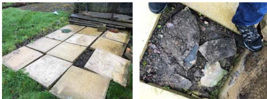
Photograph 5 and 6—Concrete flags adjacent to outbuildings
