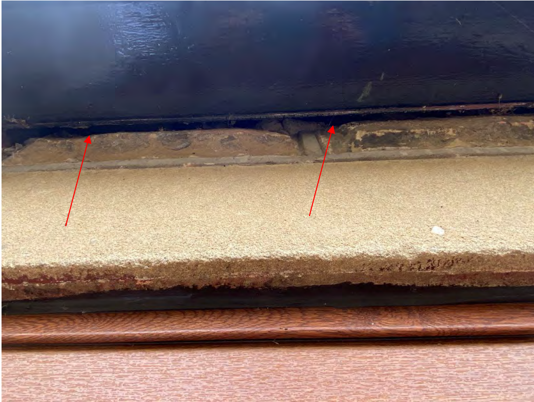
Photo 3. Potential bat roost feature at eaves on west side of porch
