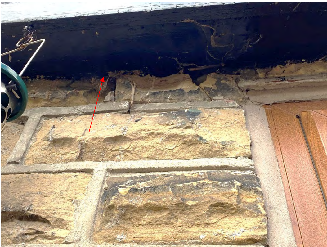
Photo 4. Potential bat roost feature (and bird droppings) at eaves on east side of porch
