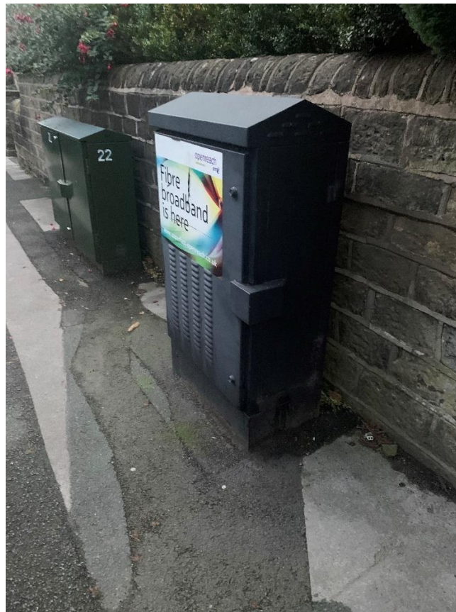
Figure 7 - BT Openreach Exchange Unit adjacent boundary wall
