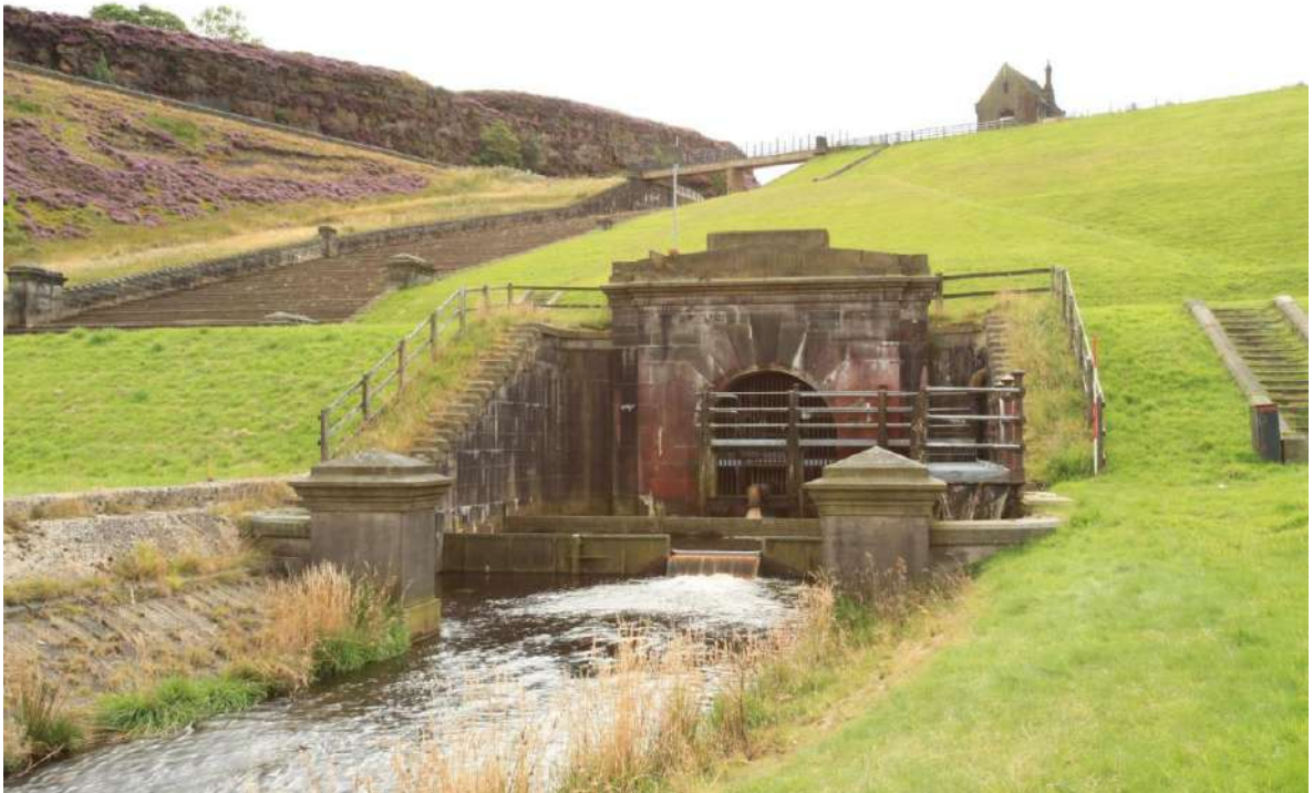
Figure 5: Bottom Outlet at Butterley Reservoir
