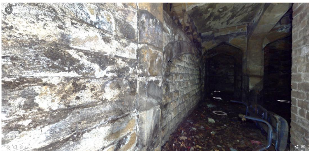
Plate 30: Blocked archway in north wall of subway area (screenshot from 3D model provided by client)
