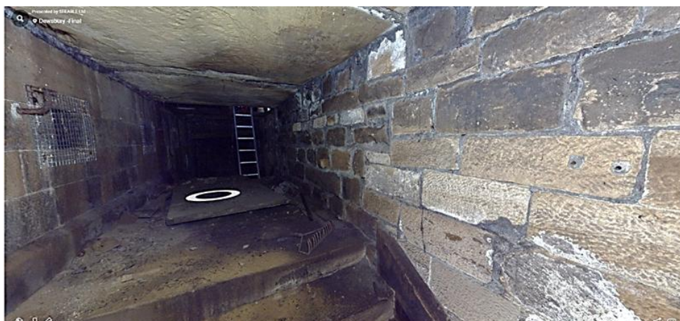
Plate 27: Entrance to subway on Platform 2, showing change in fabric on west wall (screenshot from 3D model provided by client)
