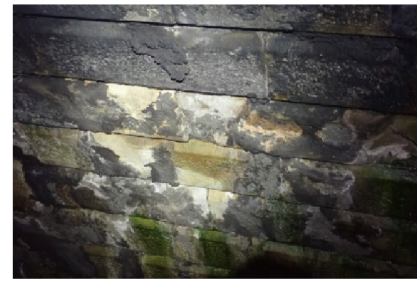
Photo 3: Defect 8 - Spalled Masonry
