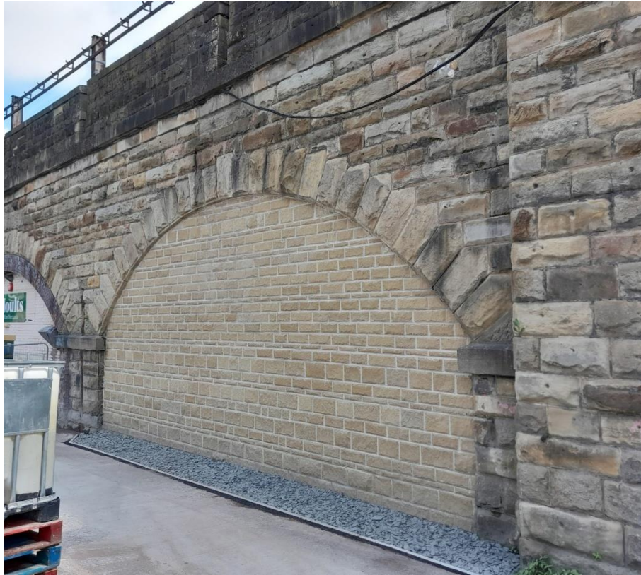
Insert 2 Use of Crosland Hill sandstone for arch infill facing on Huddersfield Viaduct (MVL3/92), evidencing appearance against existing historic stonework of similar composition to Wood Lane Overbridge (MDL1/23).
