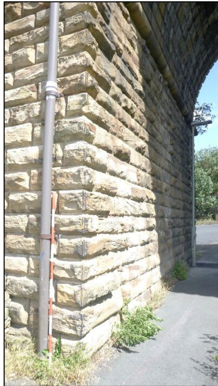
Plate 10: Tooled margin on edge of pier of Span 6 with 2m scale. View facing north-east (0485.JPG)
