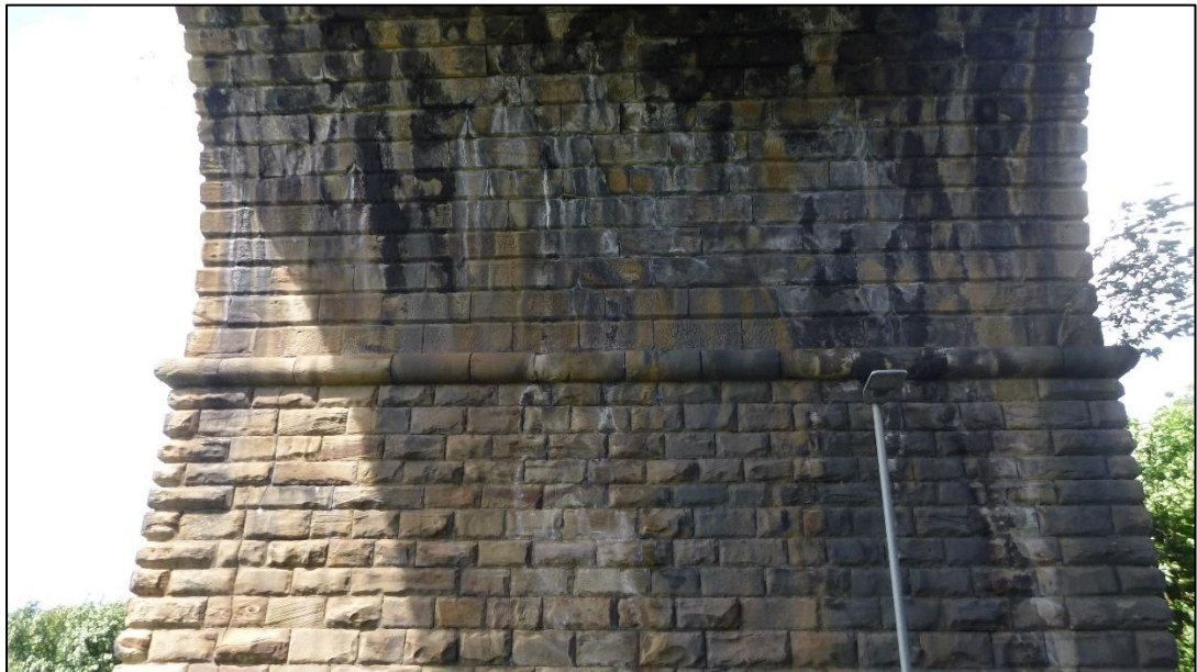
Plate 14: Moulded impost band above northern pier of Span 6. View facing north (0488.JPG)
