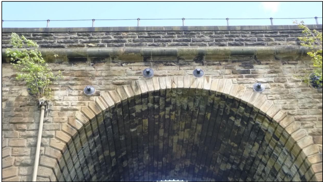
Plate 8: Voussoirs, iron supports, moulded string-course and parapet above Span 8. View facing east (0479.JPG)
