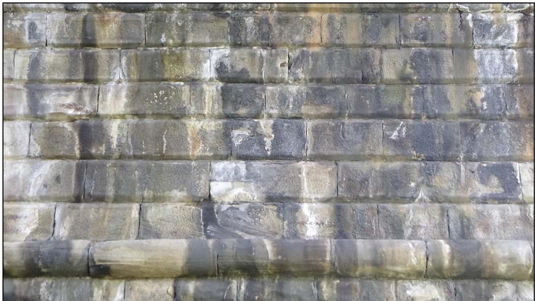
Plate 15: Rusticated stone forming underside of arch of Span 6. View facing north (0494.JPG)
