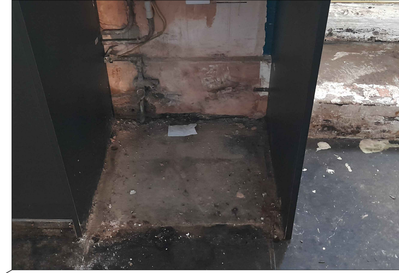
damp walls & floor to kitchen washing machine area
