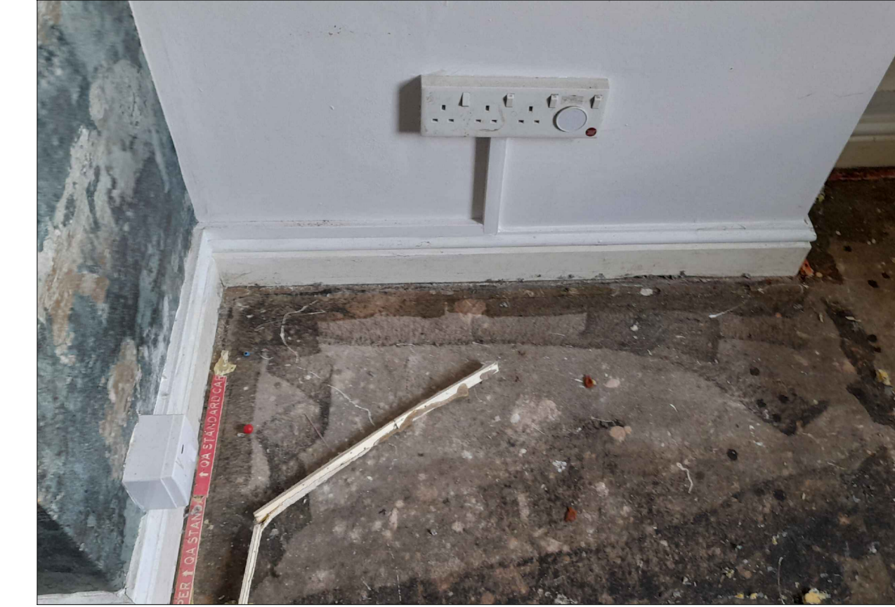
damp walls & floor in lounge
