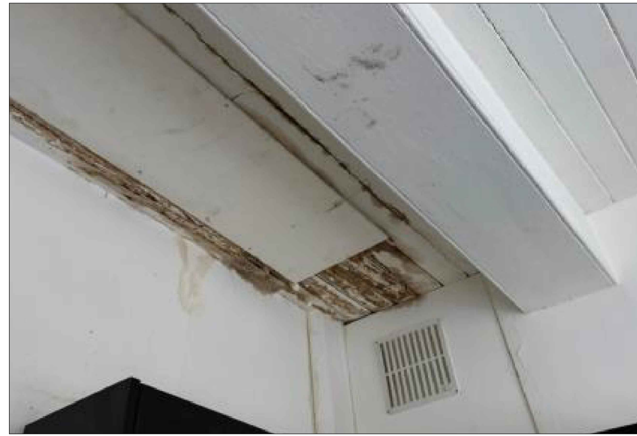
water damaged timber ceiling boards in kitchen
