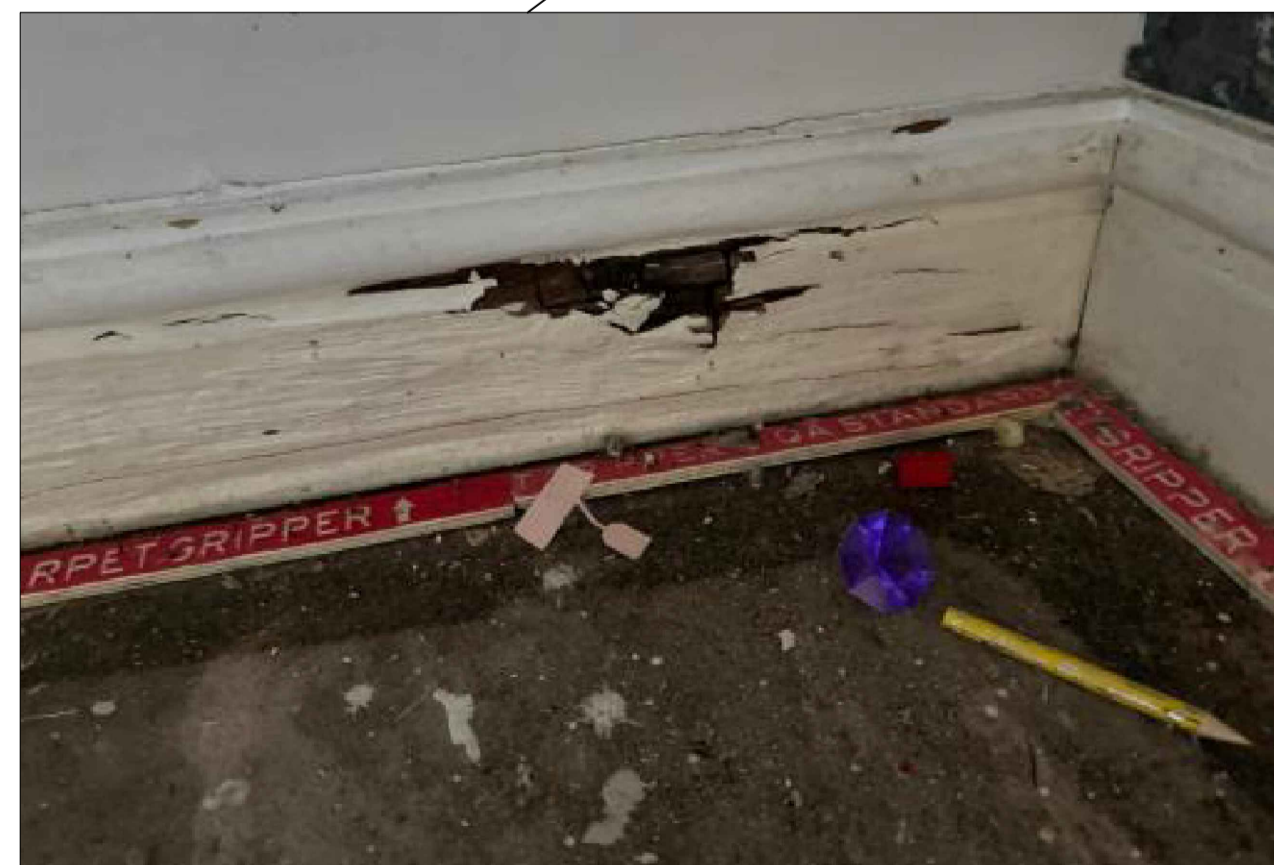
damp walls & floor - wet / dry rot to timber skirting boards in lounge
