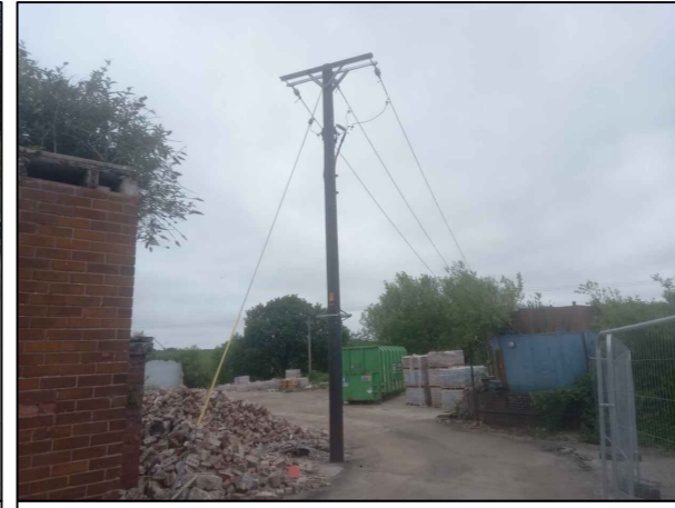
5. Newly constructed overhead cables and wooden pole, located in close proximity to former AST and sub-station.
