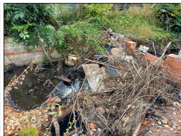
9. View of surface water culvert with discarded containers.
