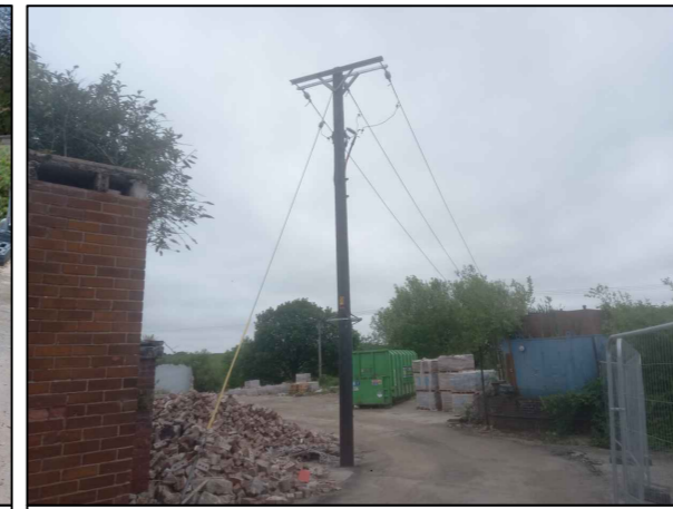
5. Newly constructed overhead cables and wooden pole, located in close proximity to former AST and sub-station.
