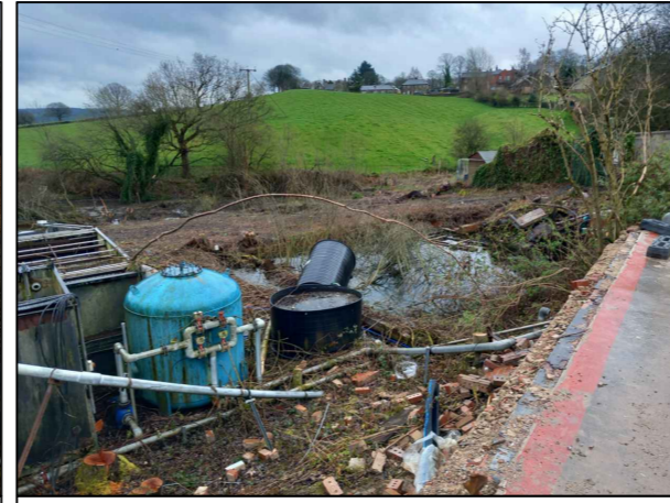
4. Evidence of former brick lined mill pond and adjacent structures prior to backfilling / clearance.
