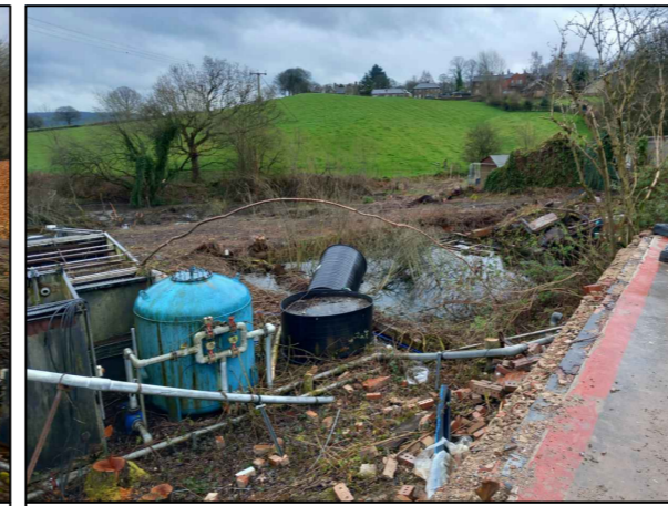
4. Evidence of former brick lined mill pond and adjacent structures prior to backfilling / clearance.
