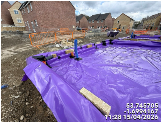
Photo 5 Multiple sealed service entries
