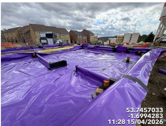
Photo 4 DPM / gas membrane used as a gas resistant DPC
