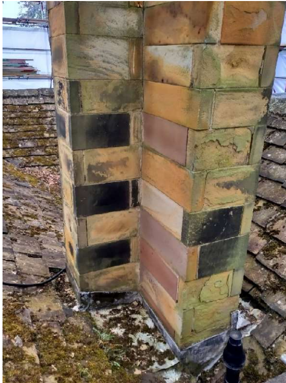
Photo 9 – Stack S3 from North (Base section) – Note heavy weathering and delamination of stonework
