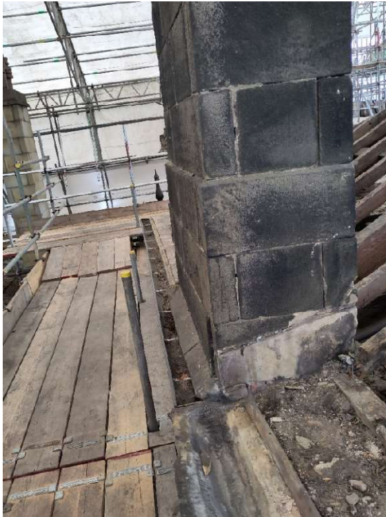
Photo 23 - Stack S5 from South, low level, highly weathered and open joints.
