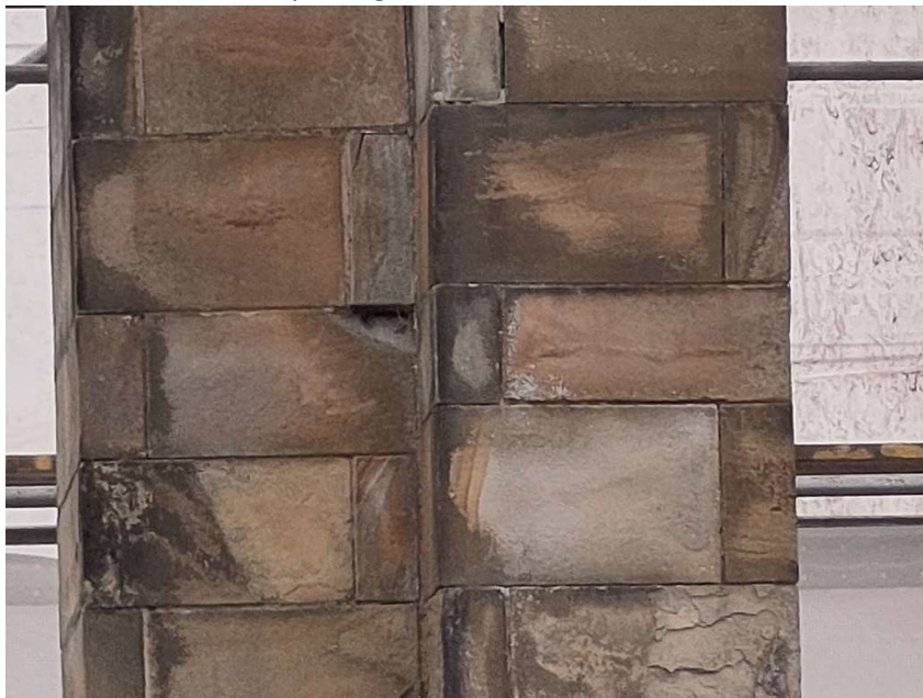
Photo 13 – Stack S3 from South, Mid Section. Heavy weathering, delamination and damage to stones.
