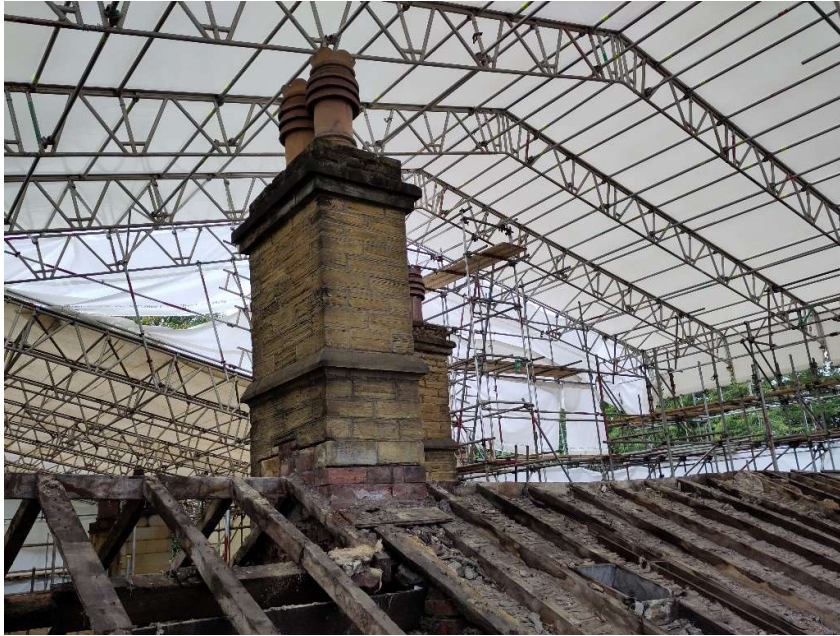
Photo 26 – Stack S7 from East
