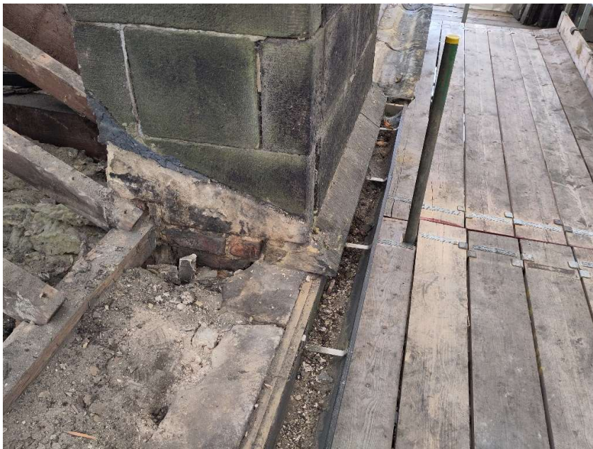
Photo 21 – Stack S5, from North West, base, highly weathered and open joints.
