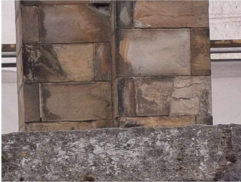
Photo 14 – Stack S3 from South, Lower Section. Heavy weathering, delamination and damage to stones.
