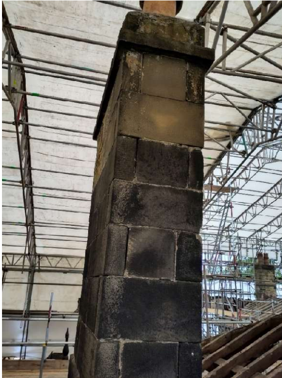
Photo 22 – Stack S5 from South, high level, highly weathered and open joints.
