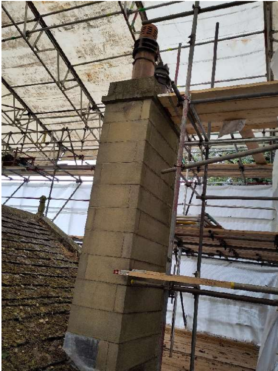
Photo 3 – Stack S1 from North, open joint to top course
