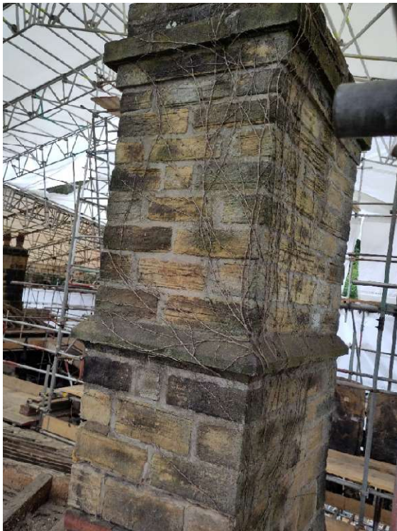
Photo 33 – Stack S9 from North East
