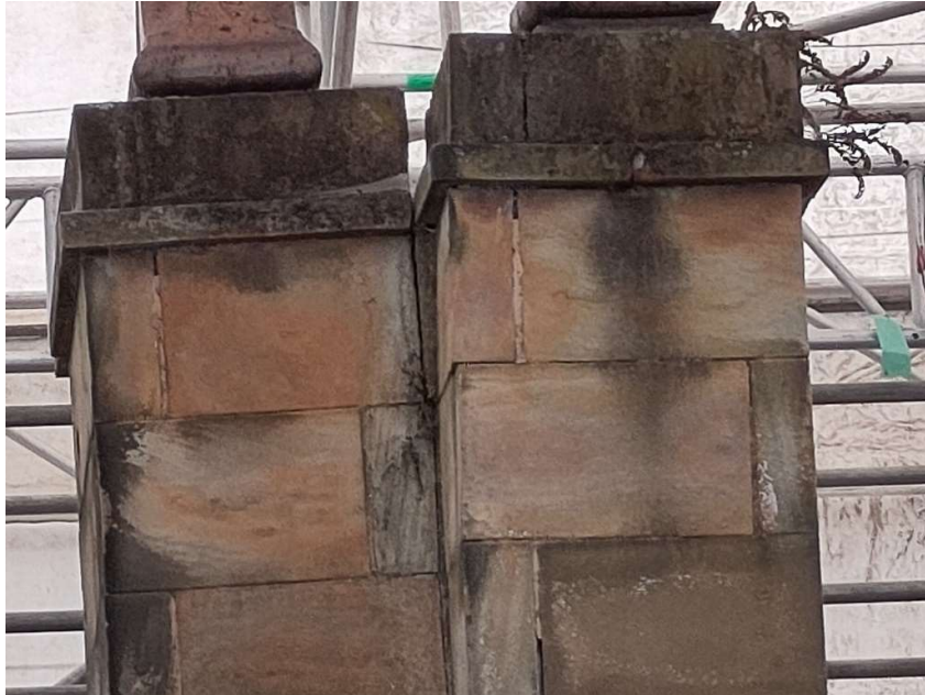
Photo 12 – Stack S3 from South, Top Section. Lean of West section of stack and sections of stack parting from one another.
