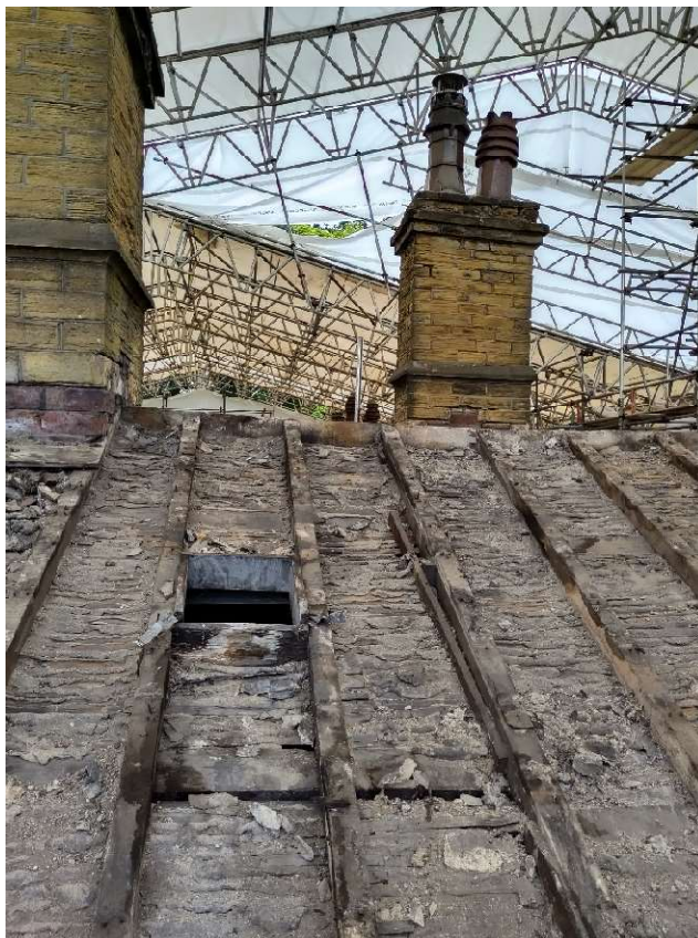
Photo 28 – Stack S8 from East. Weathered stonework above lower string course.
