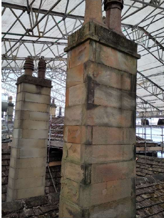
Photo 10 – Stack S3 from West (Top Section) Heavy Weathering and delamination of stones.
