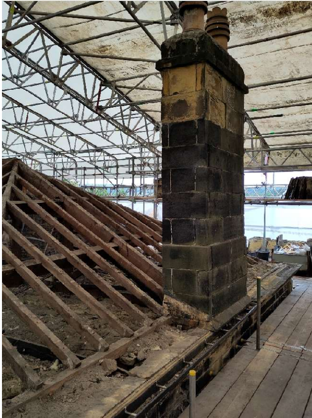
Photo 20 – Stack S5 from North West, highly weathered and delaminating stone to top courses.
