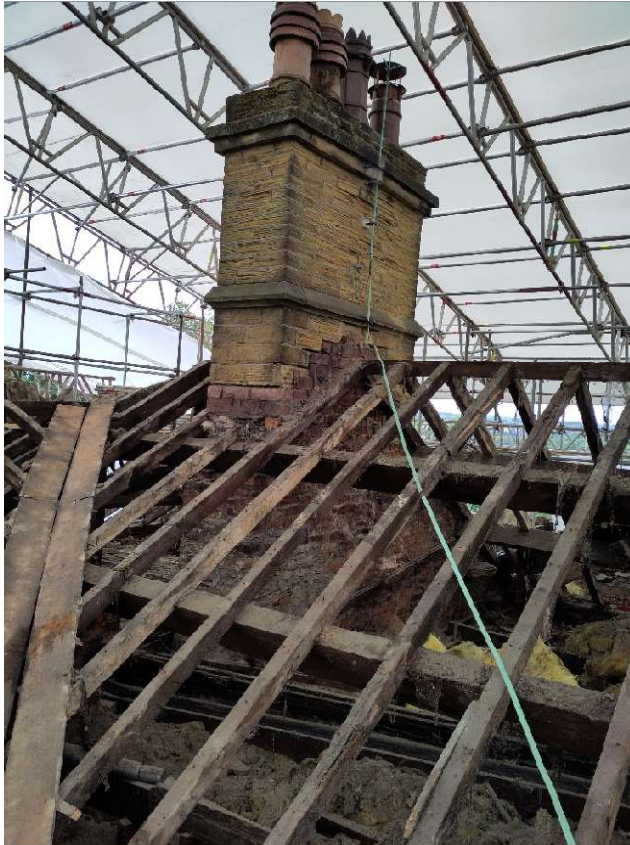
Photo 24 – Stack S6 from West. Heavily weathered stonework above lower string course
