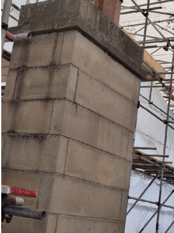
Photo 2 – Stack S1 from South, open joints to head of stack
