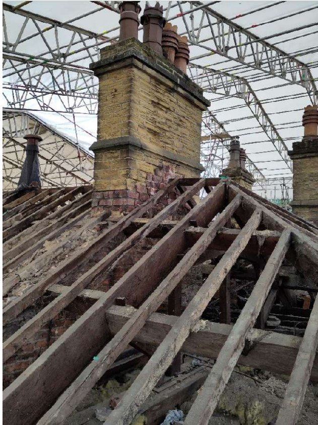
Photo 25 – Stack S6 from South East. Very heavily weathered stonework above lower string course.
