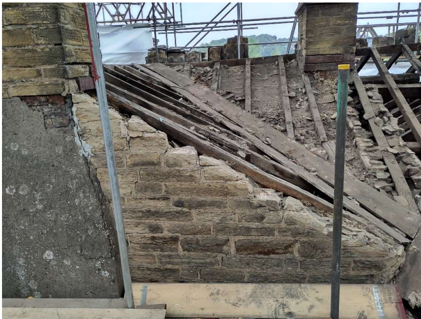
Photo 30 – Loose masonry to verge of gable peak
