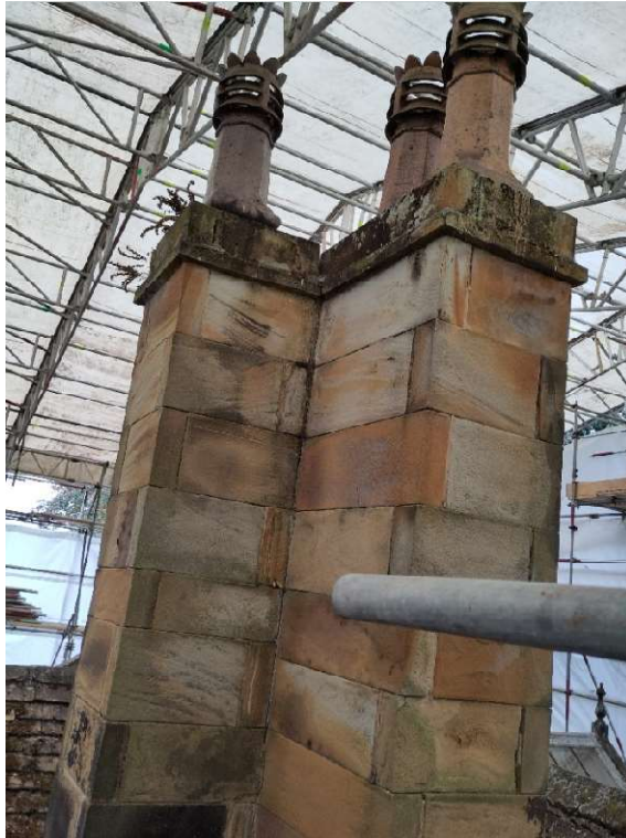
Photo 8 – Stack S3 from North (Top Section)
