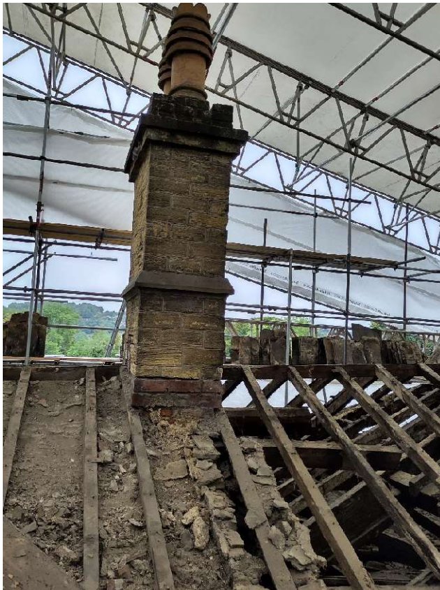
Photo 27 – Stack S7 from West. Note heavy weathering to masonry above upper string course.
