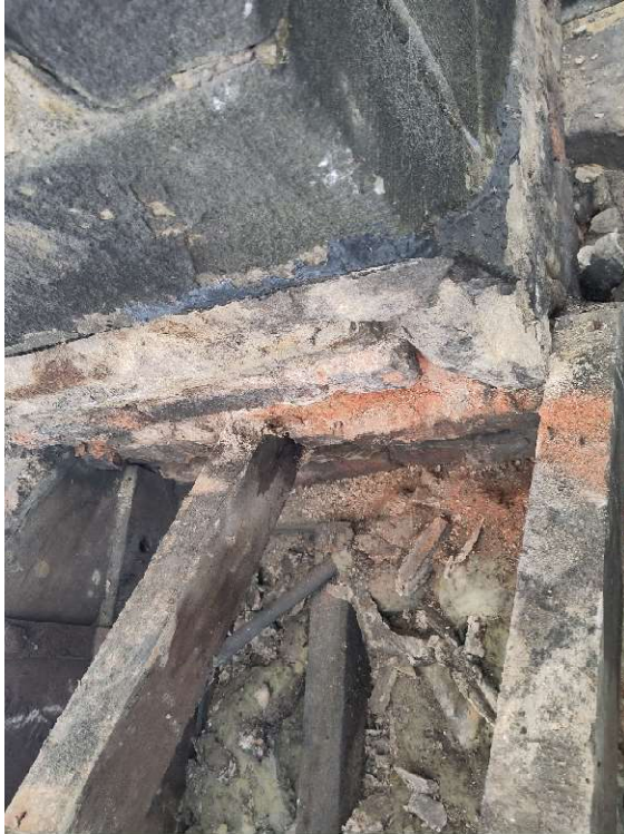
Photo 23a – Stack S5 from East. Brickwork to inner face (below original flashing line) has completely perished.
