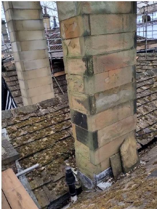
Photo 11 – Stack S3 from West (Base Section) Heavy Weathering and delamination of stones.
