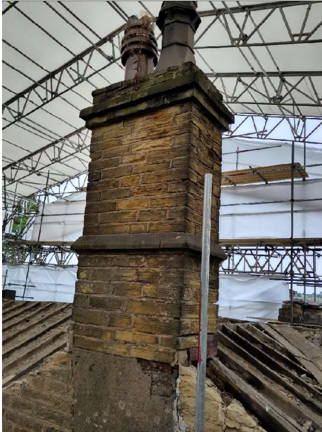
Photo 29 – Stack S8 from West. Heavily weathered stonework above lower string course. Loose masonry to verge of gable wall and rendered brickwork flue wall within gable.
