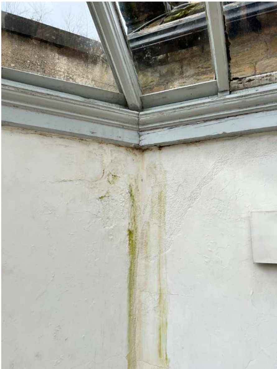
Photograph 8 - Internal water ingress damage
