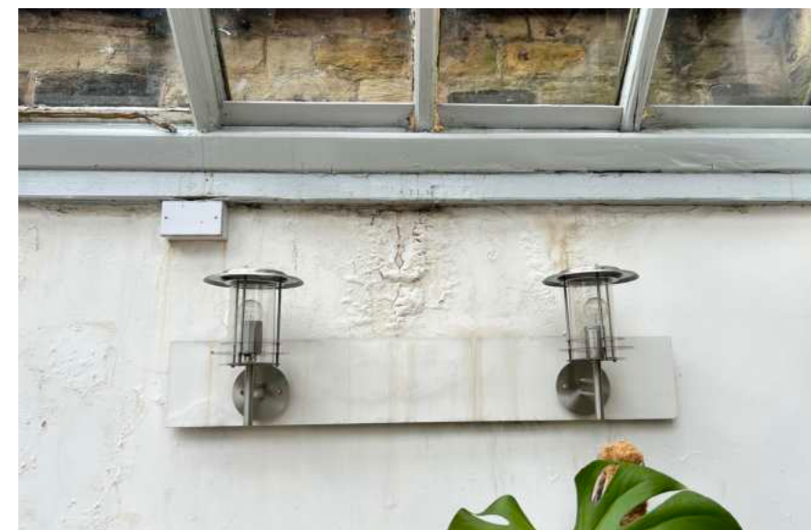
Photograph 3 - Internal back wall showing water damage
