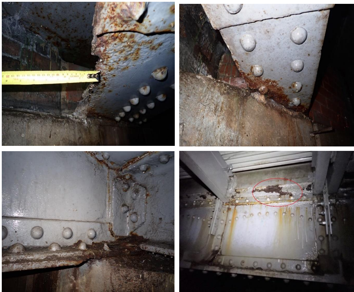
Insert 1-2 Examples of corrosion, including evidence of section loss and loss of thickness, on steel girders of MDL1/24 Jack Lane (Network Rail, 2024).
