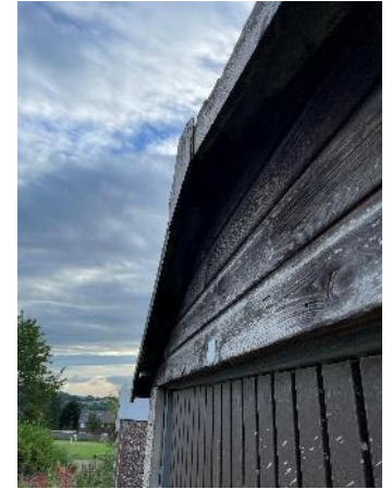
Sealed fixtures on B1
