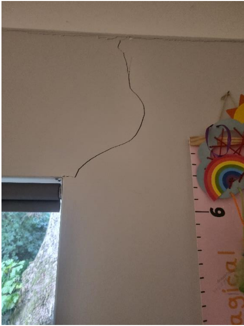
Diagonal cracking to front wall of front left-hand bedroom
