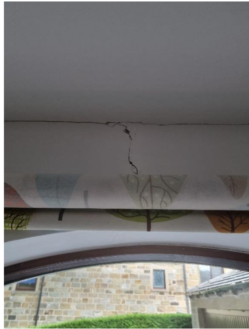
Vertical cracking to front wall of front left-hand bedroom
