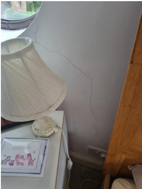
Diagonal cracking to left-hand wall of rear left-hand bedroom
