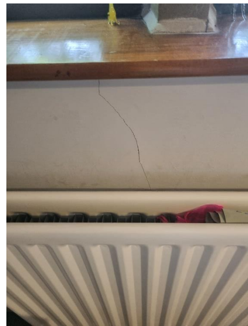
Vertical cracking to front wall of front left-hand bedroom
