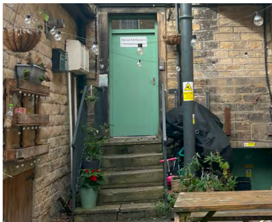
Photograph of existing rear courtyard showing entrance to existing apartments at first floor level
