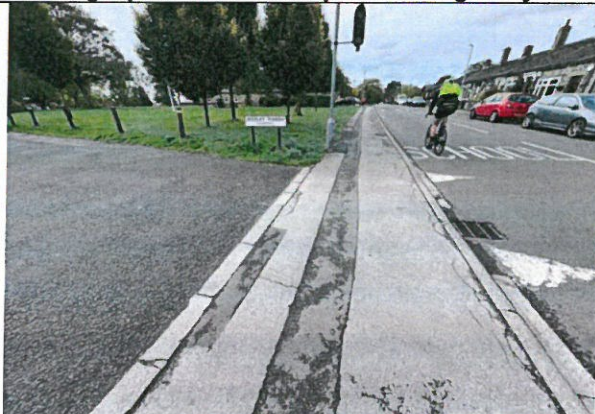
Chainage 0 – Scarring / reinstatements in footway. Cracks in several delineation kerbs to rear of footway
