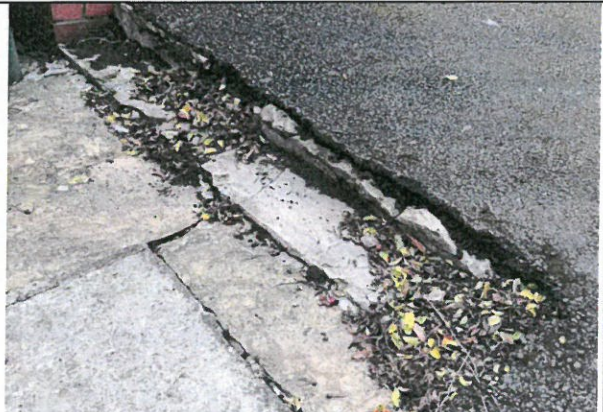
Chainage 42.8 to 44.6 – Slight collapse at back of carriageway adjacent to 'Thornfield'
