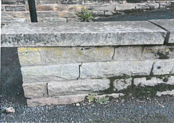
Chainage 7 – Start of pedestrian ramp. Slight crack in wall
