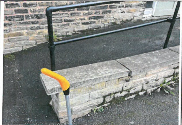
Chainage 7 – Start of pedestrian ramp. Slight crack in wall, first two coping stones loose, handrail in good condition
