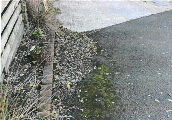
Chainage 37.6 – Start of access to 'Thornfield'. Area of surface course de-bonding adjacent to driveway
