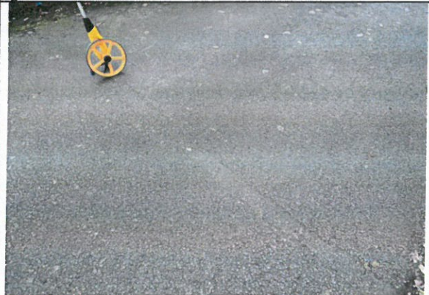
Chainage 49.6 – Scar across full width of carriageway
