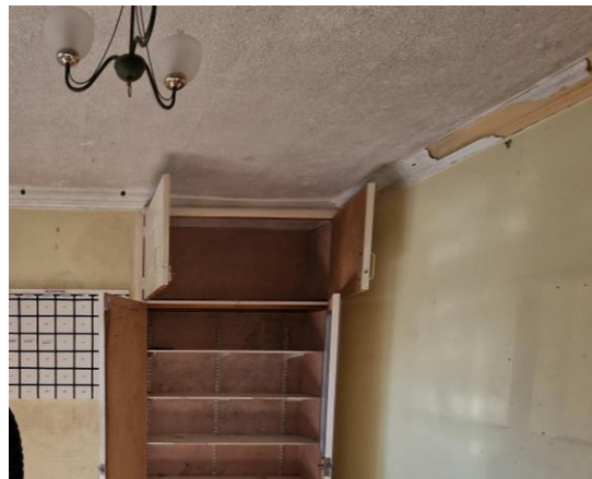
Timber coping on the right side of the image seen with paint stripping away
