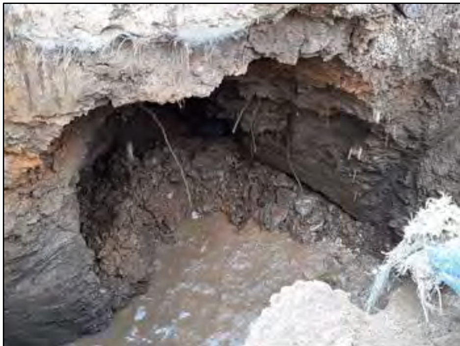
Figure 7.5.1 – Void Identified in TT204B (1.5mbgl and 3.0mbgl).
