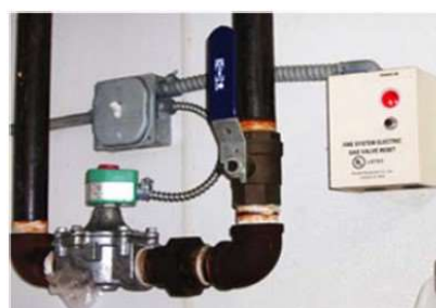
Fig No. 11. Example of automatic gas isolation valve
