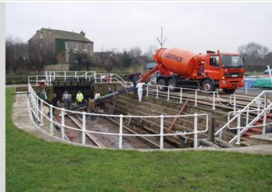
16. Reinforced concrete laid over original stonework at base of dry dock. Railings and paving slabs installed around perimeter.
