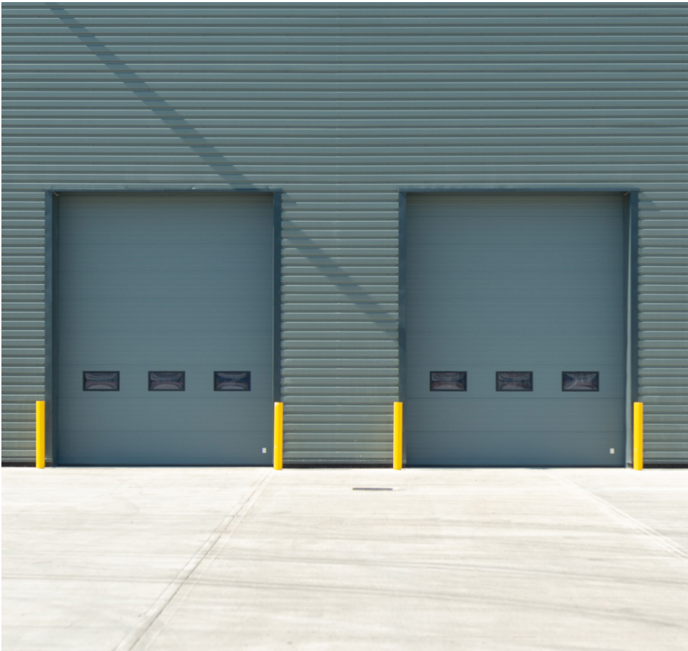
Above - Sectional overhead doors
