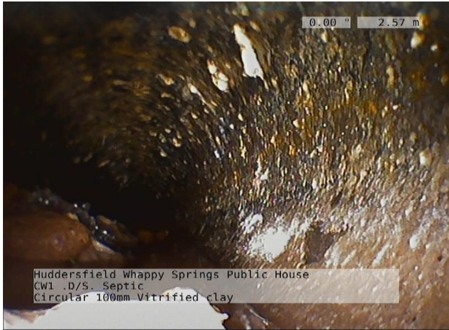
CW1-DSeptic-1-27853.jpg, 00:00:39, 2.57 m Settled deposits, other, 15% cross-sectional area loss, Rags
