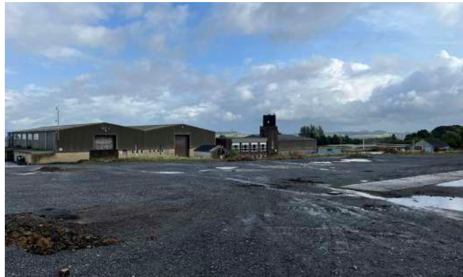
2. View of the existing buildings to be demolished in the eastern part of the site.
