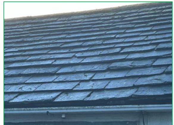
Showing gaps under the slates on the north elevation of the house
