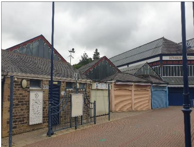
Plate 9. The gents toilet block in the centre of the Site. With adjacent trader stalls.
