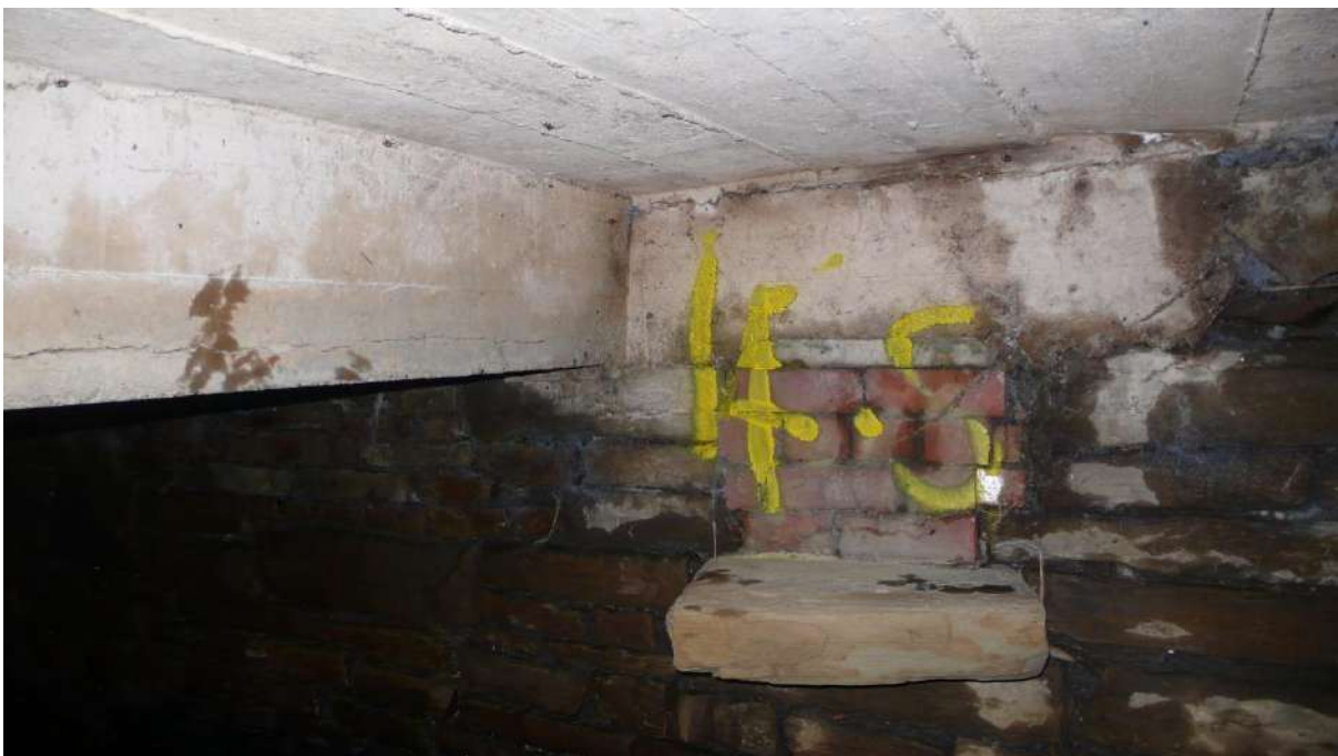
Photograph 32 11.5m RHS ledge sticking out of wall. Note crack to side of reinforced concrete beam.
