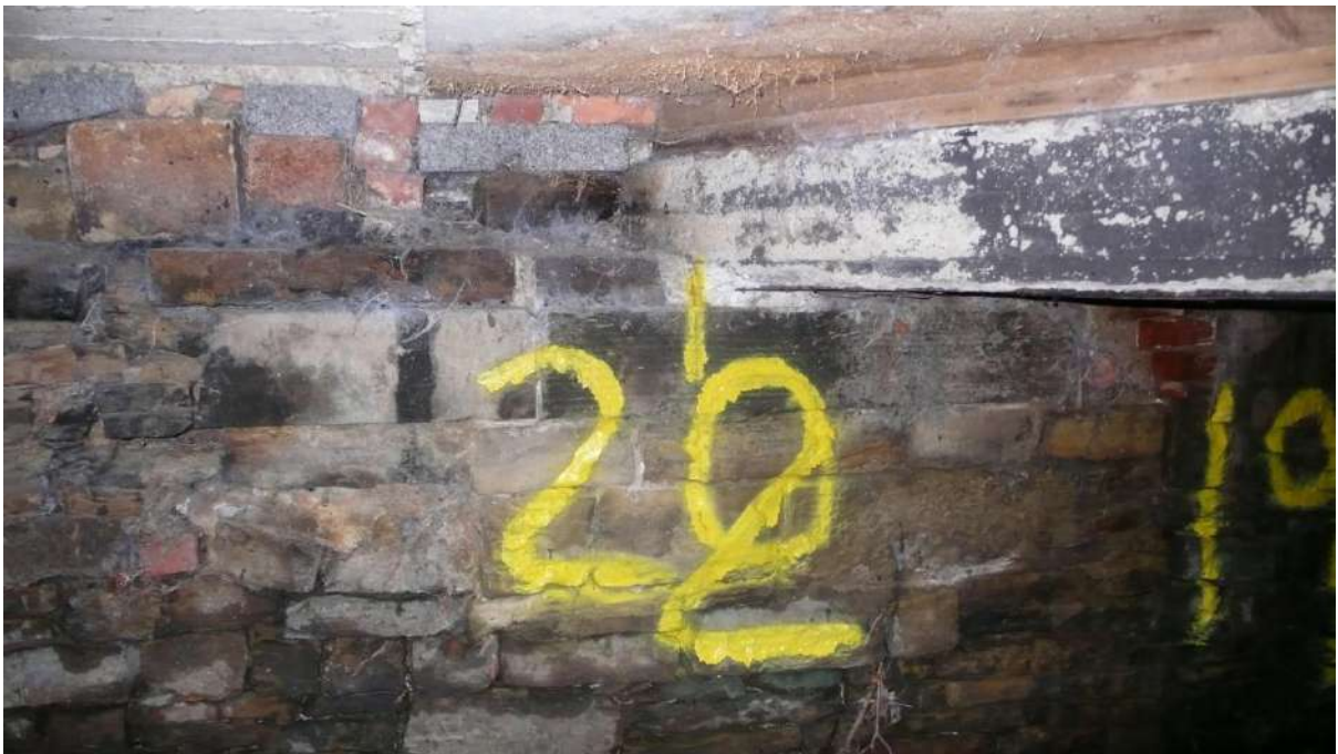
Photograph 28 22m RHS corroded RSJ with timber pack supporting soffit
