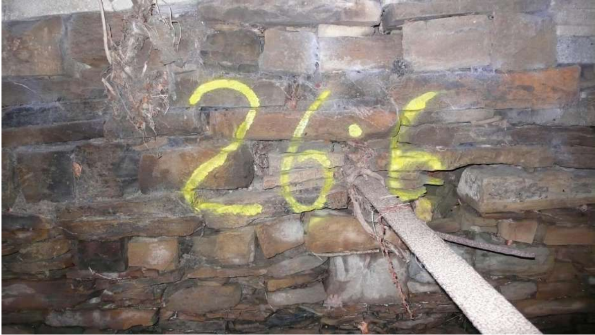
Photograph 23 26.6m LHS square-on view of corroded steel strut showing poor condition of supporting wall.
