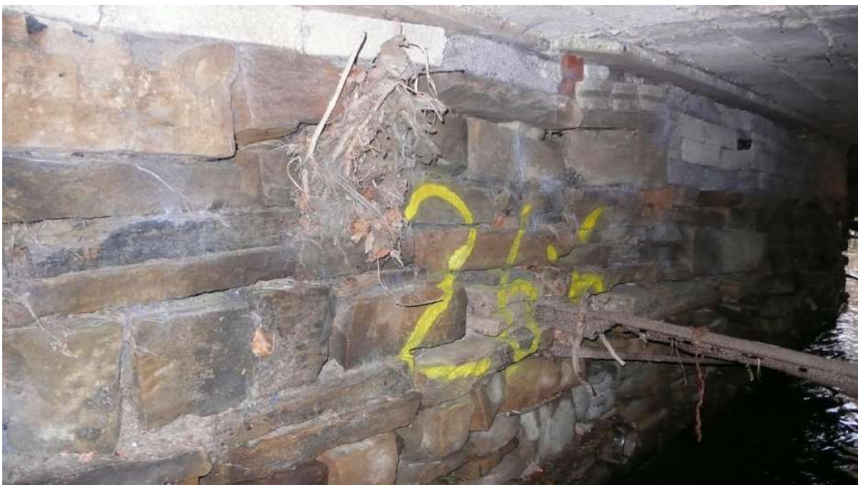
Photograph 22 26.6m LHS. Supporting wall in poor condition. Corroded steel strut across culvert at mid height. Exit (downstream) visible of RHS.
