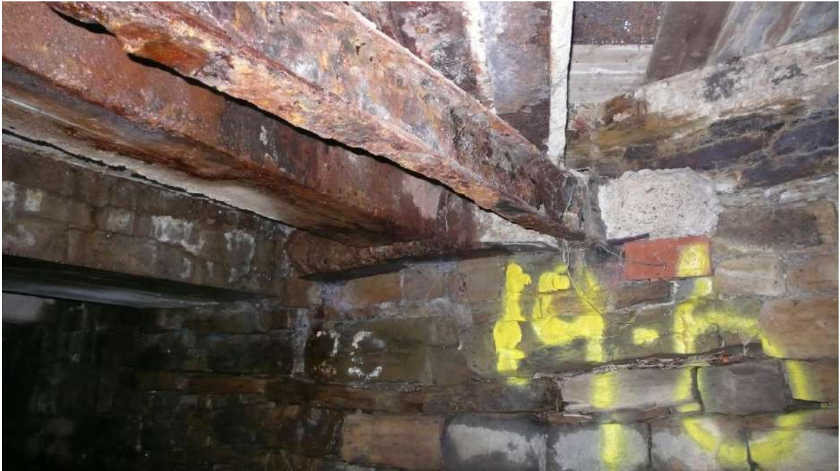
Photograph 19 19.6m LHS close-up of rusted RSJ and other steelwork/timber soffit.
