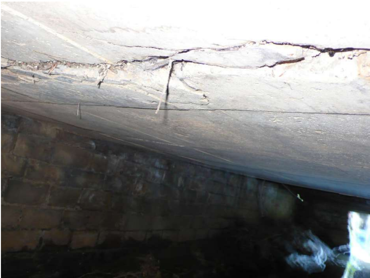
Photograph 18 18.0 approximately central. Crack and spalling of concrete soffit.
