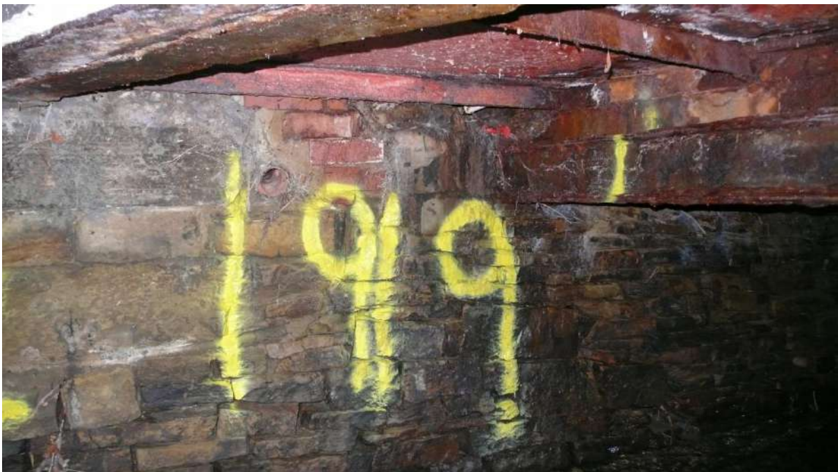
Photograph 30 19m RHS badly corroded RSJ support with additional steel members above. Badly corroded soffit support steel work ('L' members). Drainpipe through culvert wall and additional white plastic pipe (drain?) through soffit.
