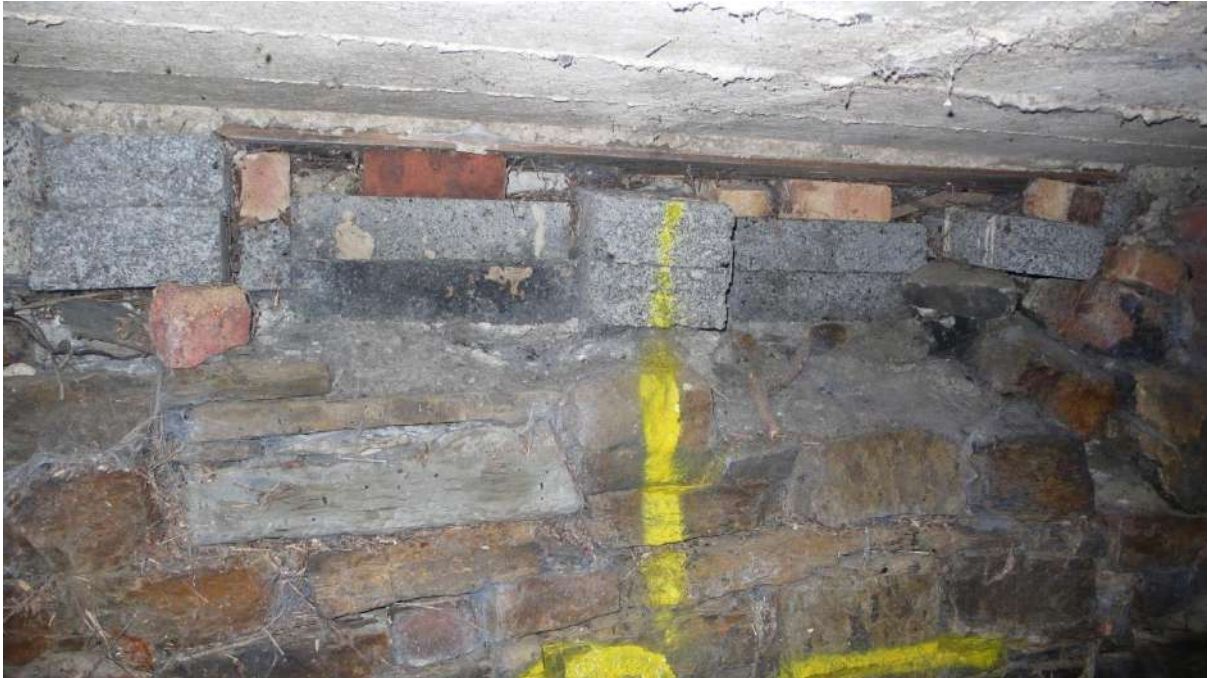
Photograph 27 25m RHS close-up of poor breezeblock and stone supporting wall.
