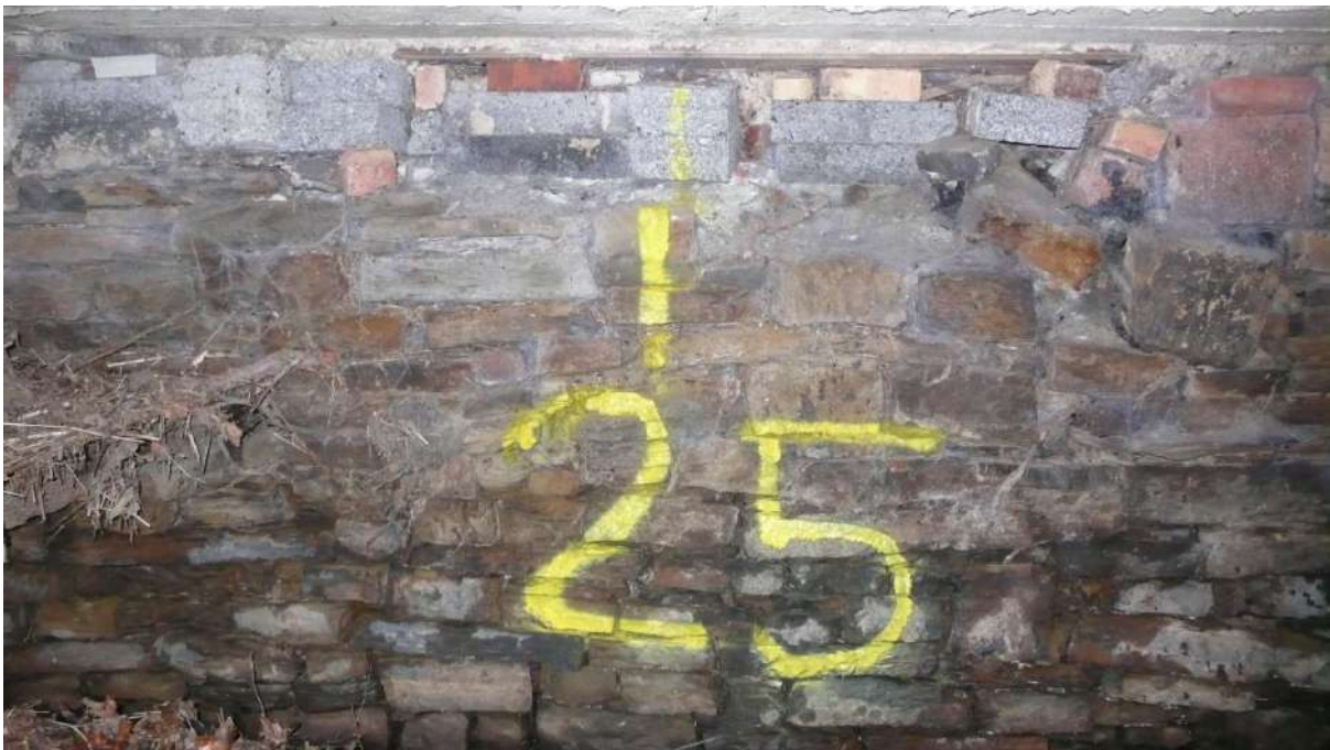
Photograph 26 25m RHS poor quality breezeblock and loose stone supporting wall.
