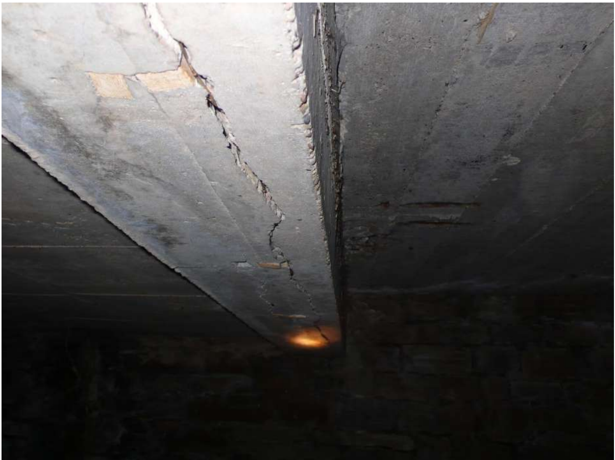
Photograph 16 17.0m approximate concrete beam showing crack to underneath and spalling to soffit.
