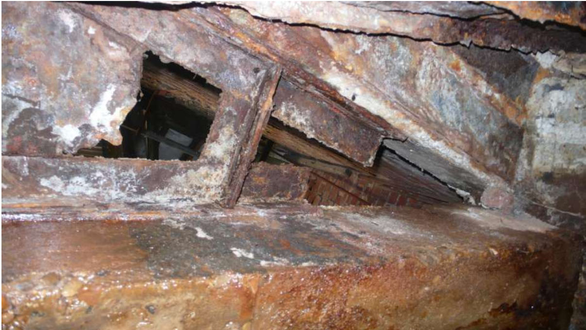
Photograph 21 19.6m LHS. Looking up through hole in culvert roof. Internal factory wall visible above.
