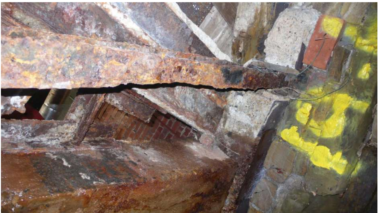
Photograph 20 19.6m LHS looking up. Rusted RSH and hole in culvert roof. Internal factory wall can be seen above.
