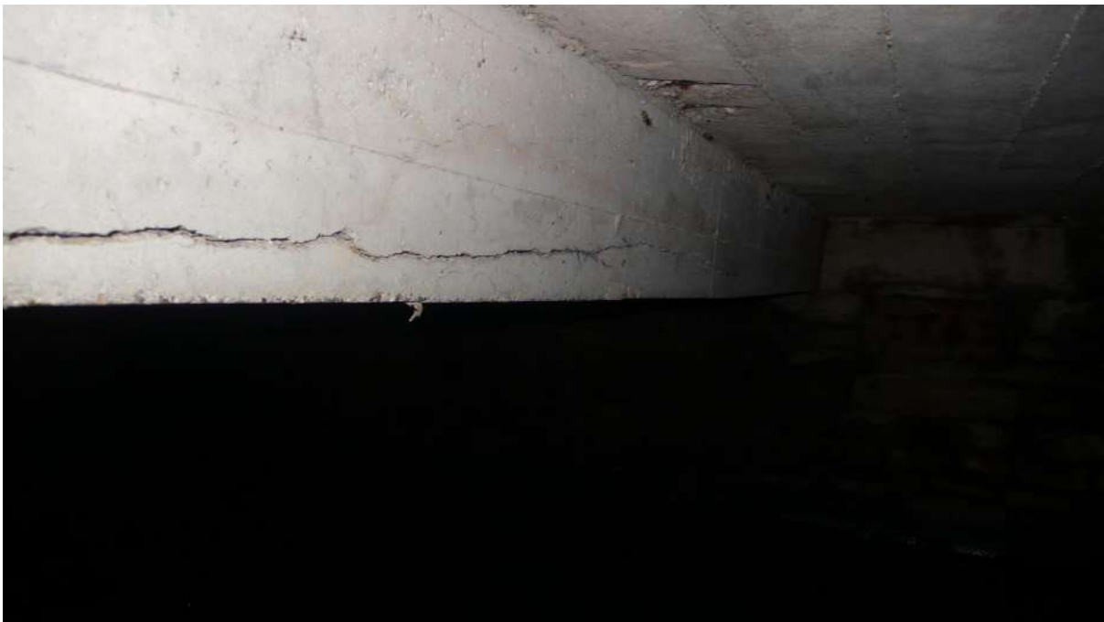
Photograph 14 14.4m LHS concrete beam showing extent of crack to upstream face of beam and spalling concrete to soffit.
