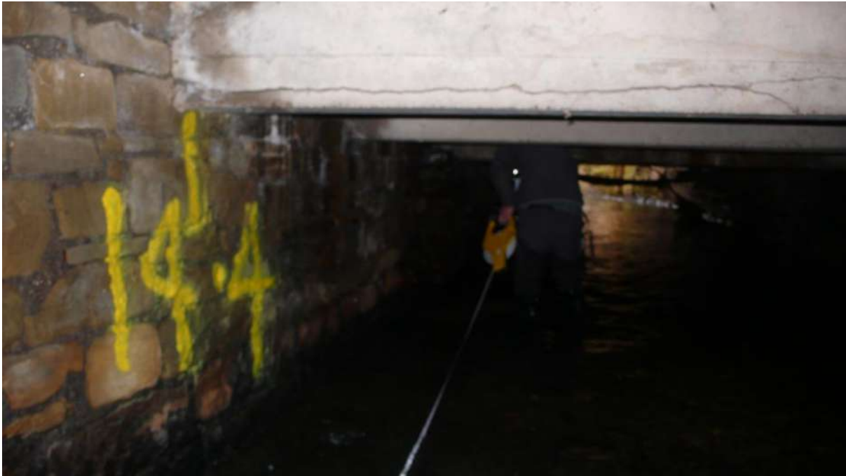
Photograph 13 14.4m LHS concrete beam showing crack to upstream face of beam.
