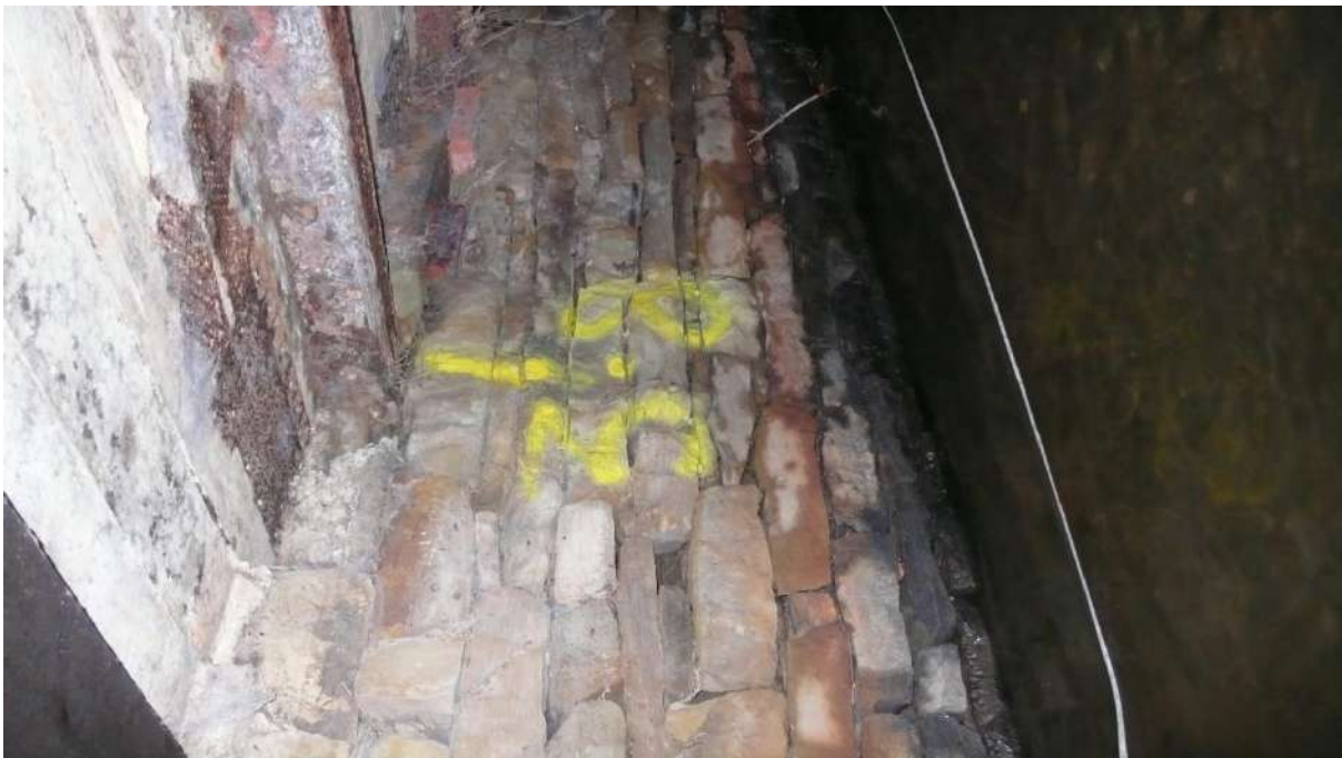
Photograph 2 3.8m LHS RSJ supporting soffit is badly corroded. Exposed rusted metal grille to soffit upstream of RSJ.
