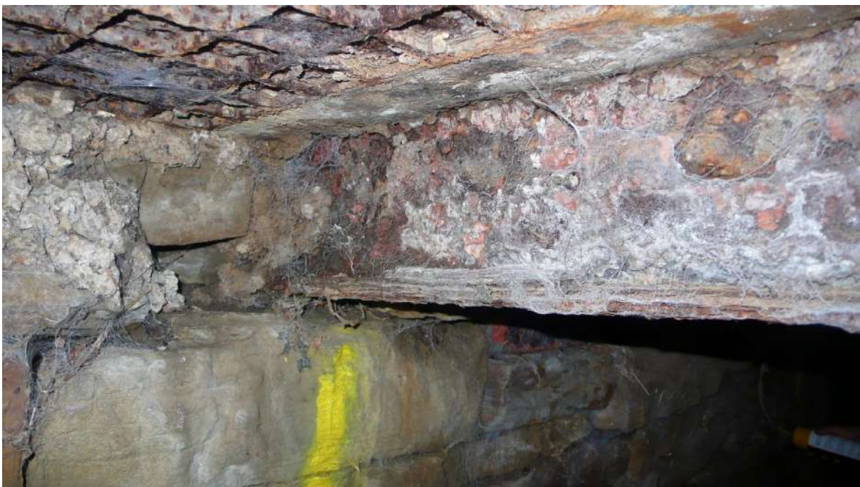
Photograph 4 3.8m LHS close-up of RSJ, metal grille to soffit, padstone and infill.
