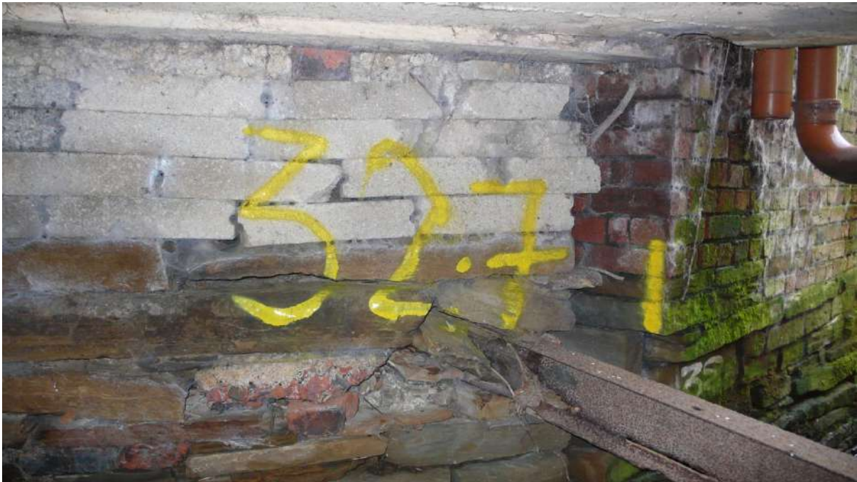
Photograph 24 32.7m LHS corroded RSJ built-in across culvert at mid height. Poor quality of supporting wall.
