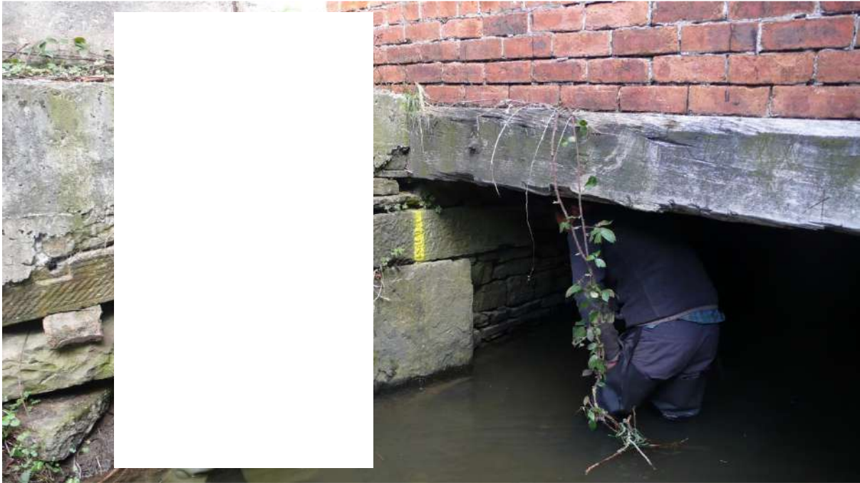
Photograph 1 Entering upstream end (SW) of culvert, chainage zero spray paint on left-hand wall (looking downstream).
