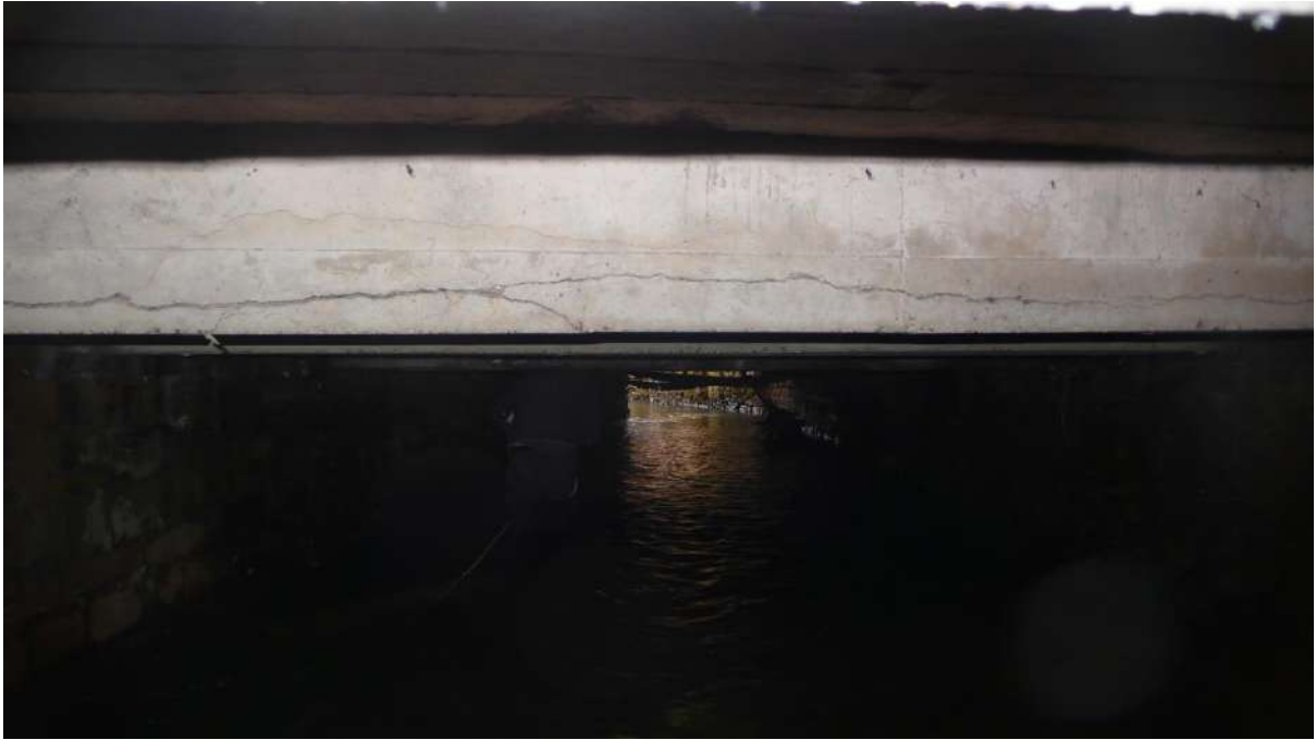
Photograph 15 14.4m centre of stream showing extent of crack to upstream face of beam.
