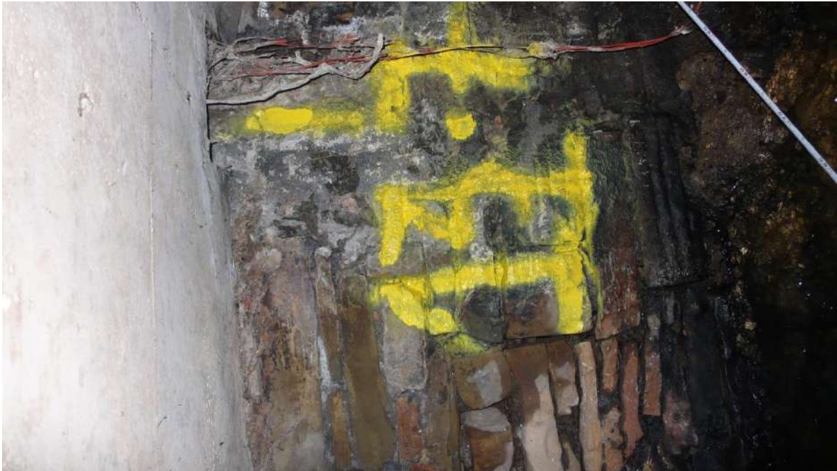
Photograph 9 11.7m LHS rectangular void through soffit.
