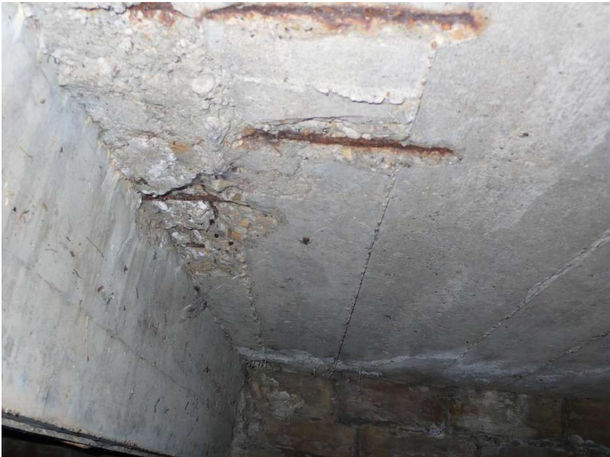
Photograph 17 17.0m approximate close-up of spalling to soffit.
