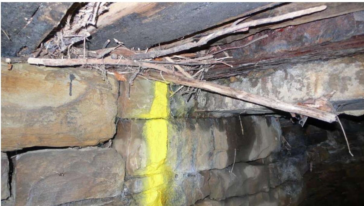
Photograph 6 5.7m LHS close-up of corroded RSJ, padstone, timber soffit formwork and trapped debris.
