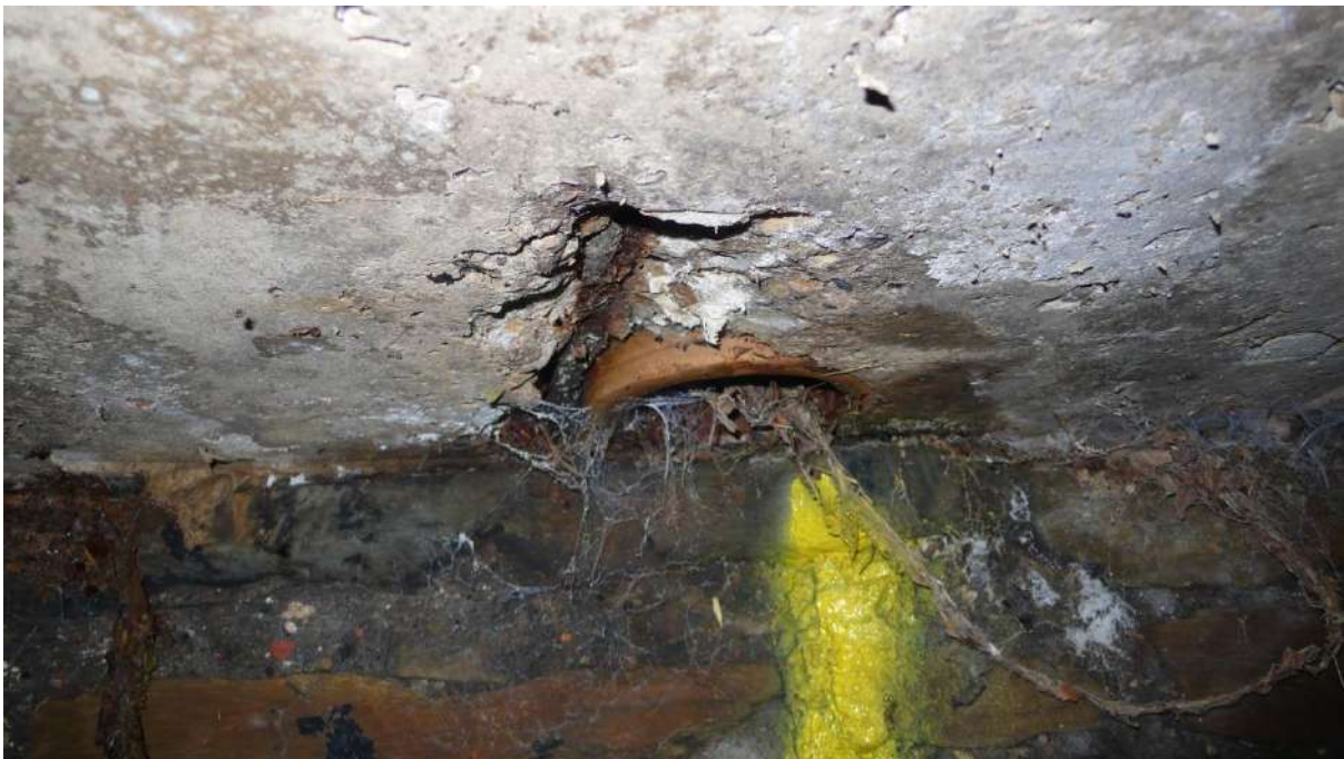
Photograph 8 10.0m LHS close-up of 4" drainpipe mostly blocked with debris/cobwebs.
