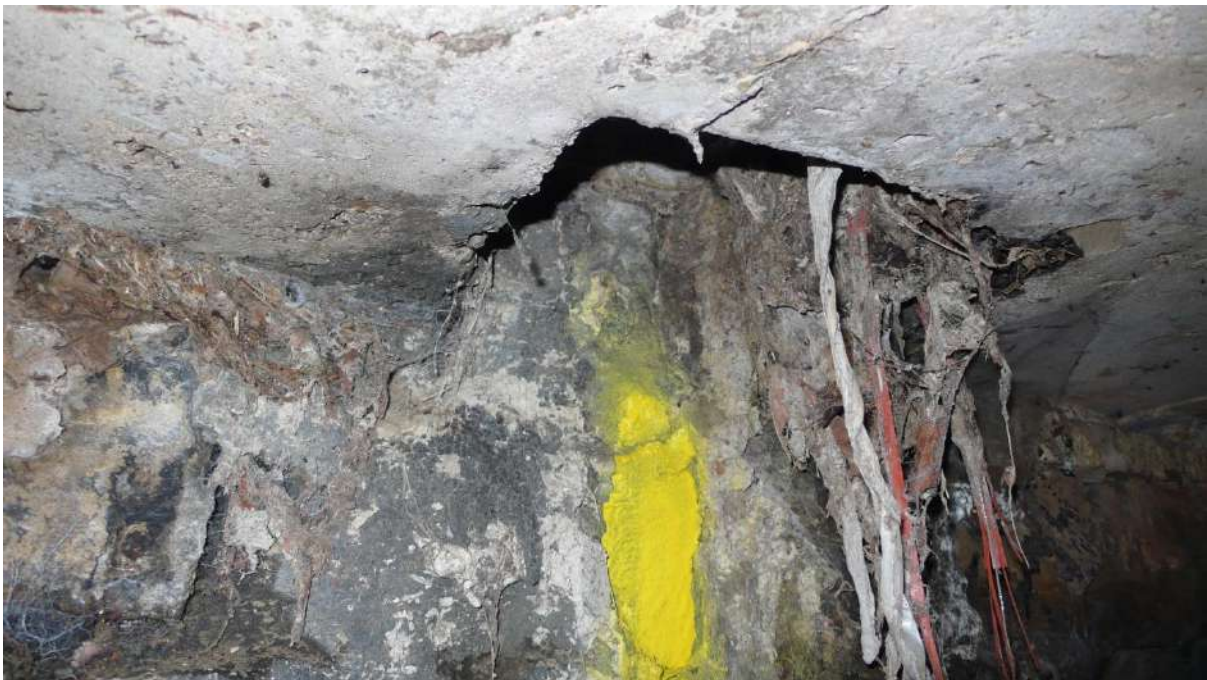
Photograph 10 11.7m LHS close-up of rectangular void through soffit showing roots/debris growing through.
