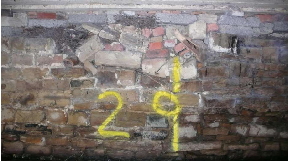
Photograph 25 29m RHS poor quality breezeblock and loose stone supporting wall. Pigeons nest.
