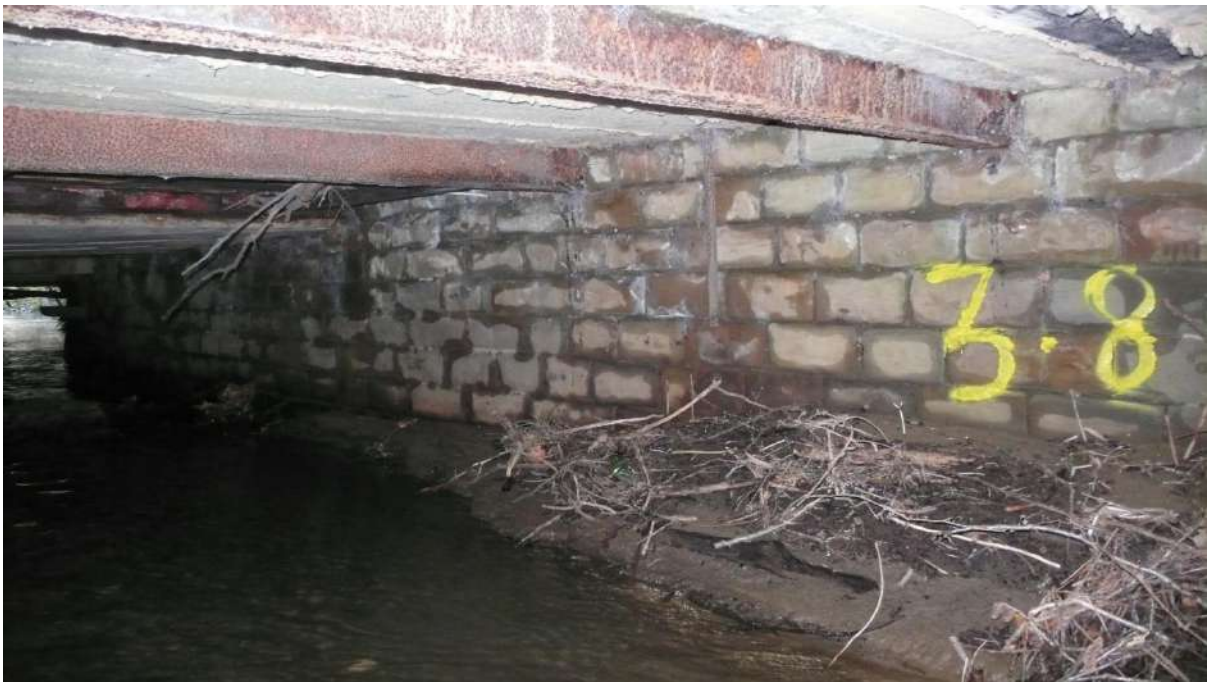
Photograph 33 3.8m RHS. Rusted RSJ. Build-up of silt and debris against right-hand wall.
