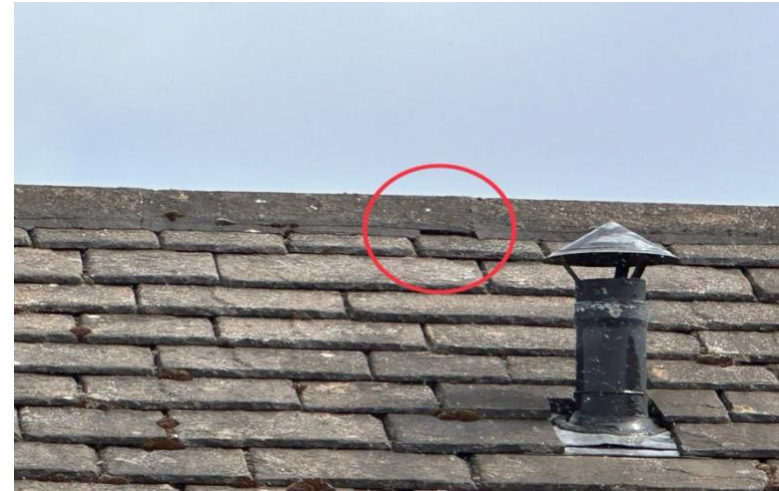
Image 6: Gap between ridge tile and slate roof tile
