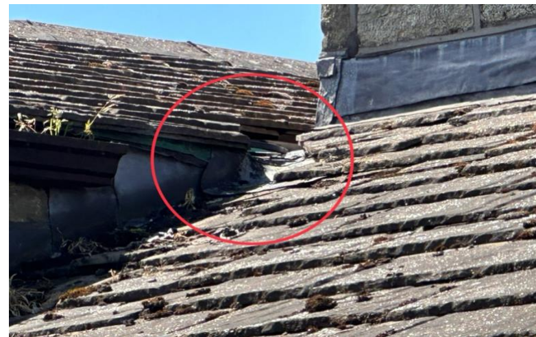
Image 16: Gaps under the slate tiles along the northeastern elevation of B1
