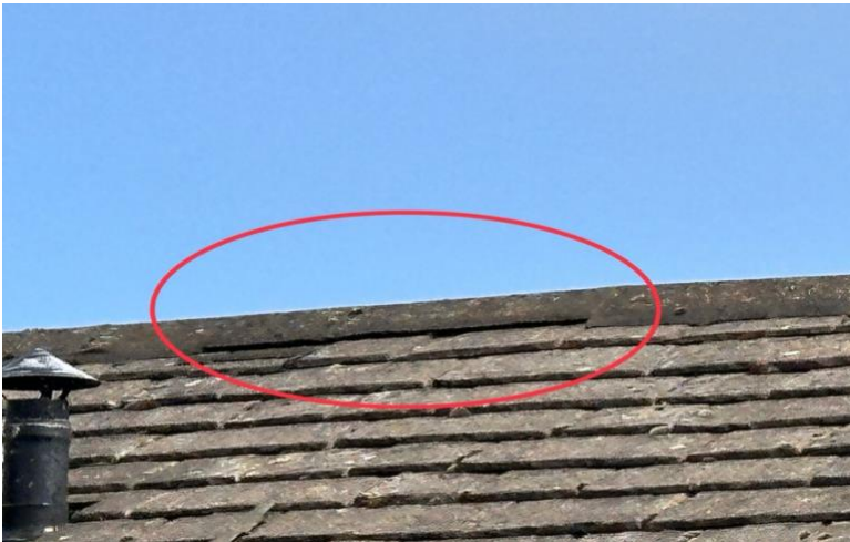
Image 7: Gap between ridge tile and slate roof tile
