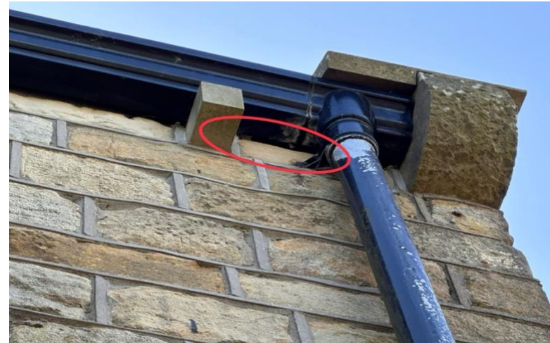
Image 14: Gap behind guttering along the northwestern elevation of B1
