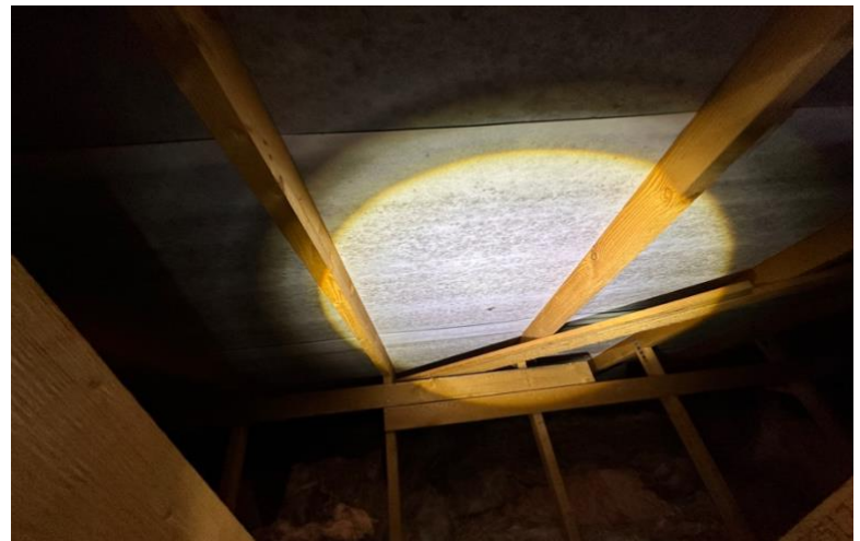
Image 32: Area of water damage to the breathable membrane within L3
