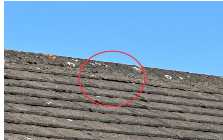
Image 8: Gap between ridge tile and slate roof tile
