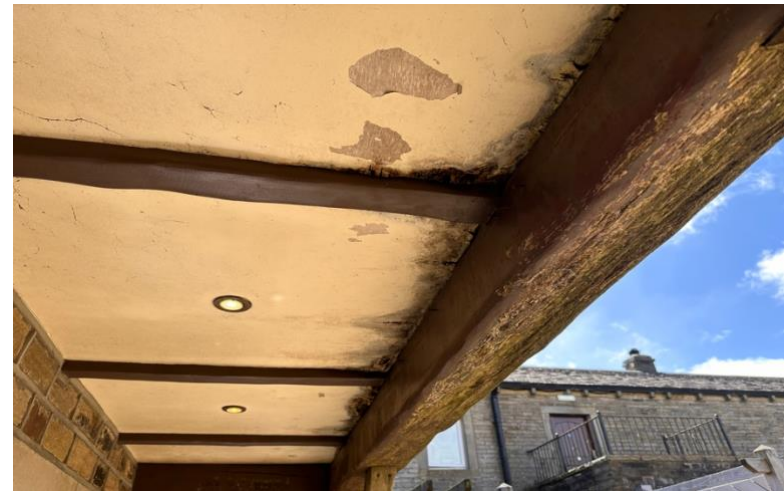
Image 12: Gaps under entrance canopy
