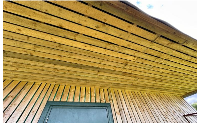
Image 38: Gaps between battens along the underside of the canopy on B3
