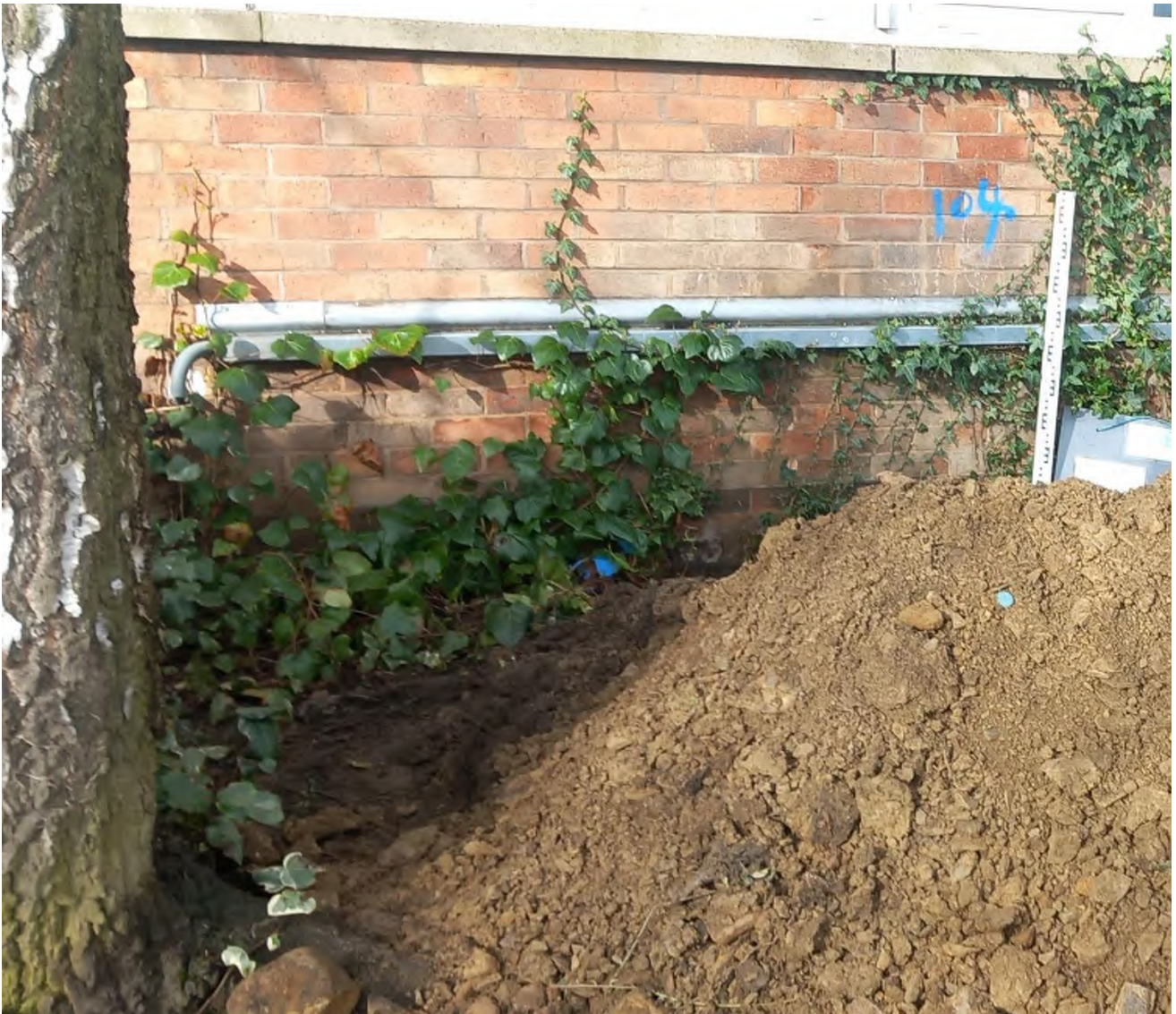
24/02/22 Photo 8 FP104. Loose made ground of reworked natural backfill below topsoil to 1.5m depth.
