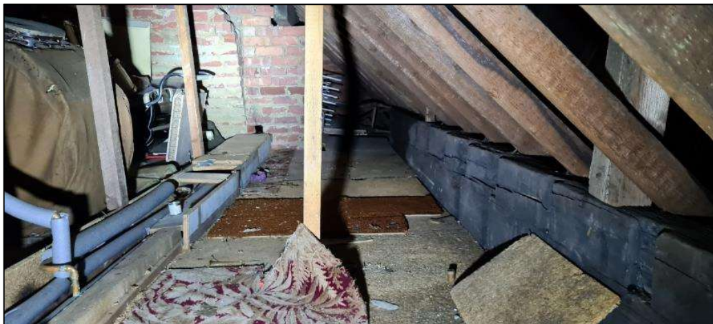
Plate 4. The void in the eaves on the east side of the building
