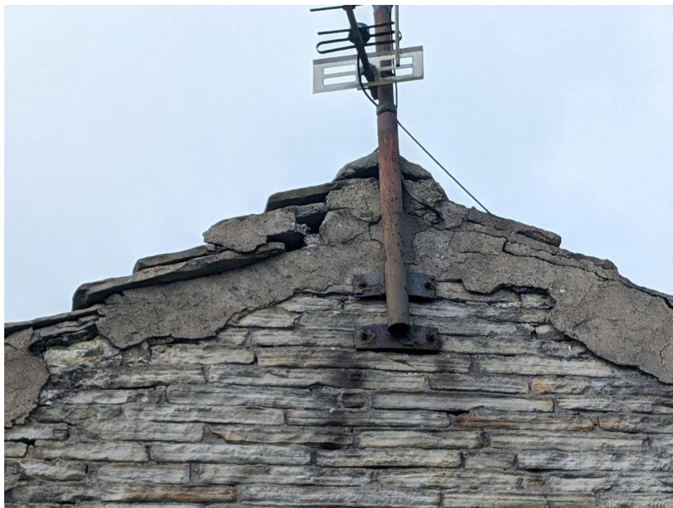
Photo 2. Gaps at ridge of dwelling (east elevation)
