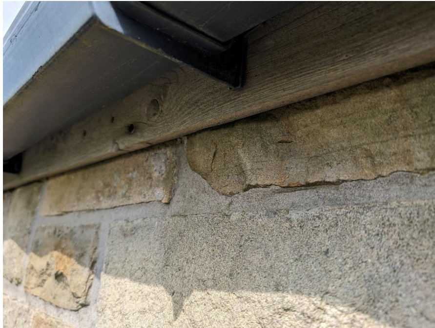
Photo 5. Gap under fascia board of dwelling (south aspect).
