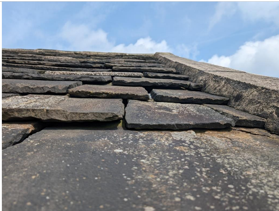
Photo 4. Numerous gaps in roof of dwelling.
