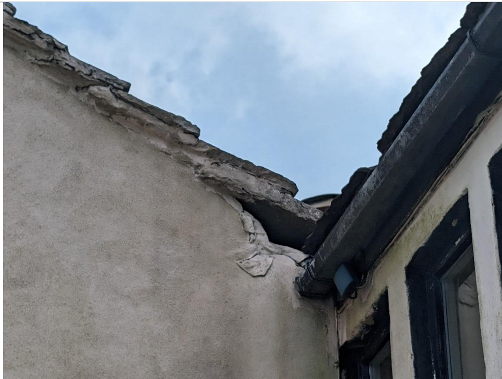
Photo 8. Large gap on corner of roof of dwelling.
