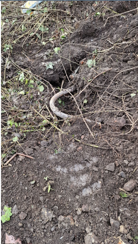
Lead pipe uncovered in TPA
