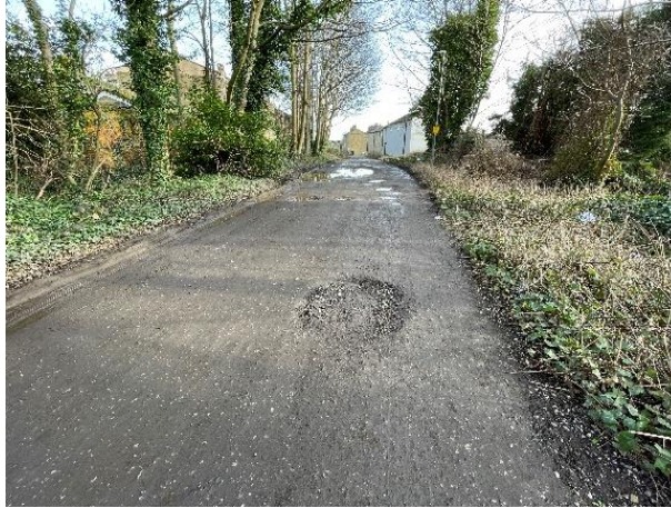
Figure 6 Artificial unvegetated, unsealed surface of Croft Street.
