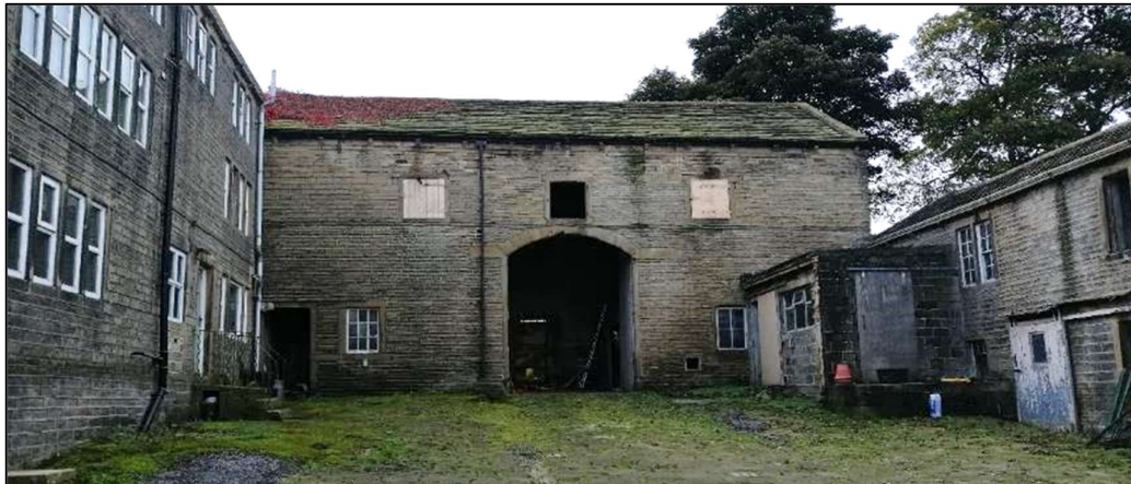
Plate 3. Front (southeast elevation) of B2, B1 on left and B3 on right
