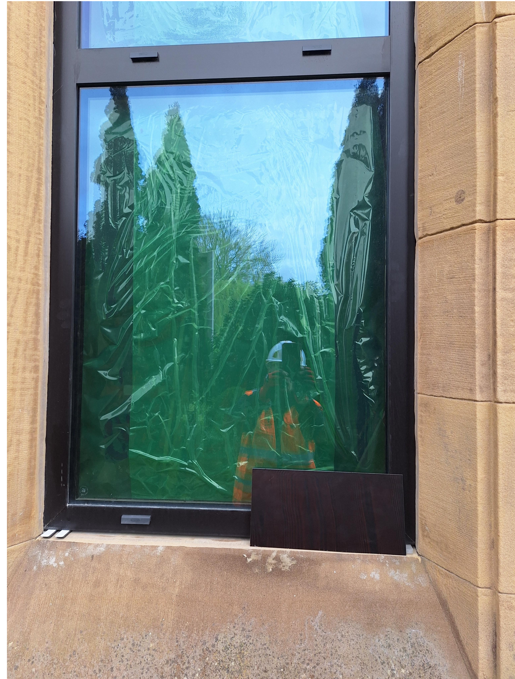
Woodgrain Ref: BWF 4 - Mahogany (Sample beside installed window)
