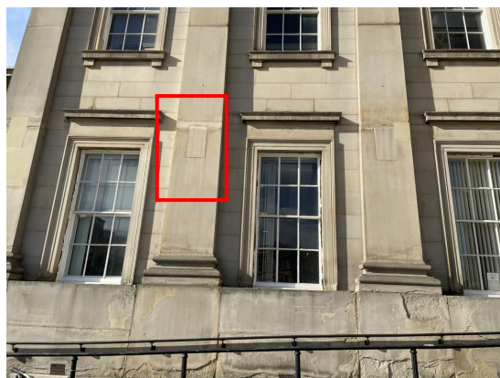
Image 13 – Markings to façade from previous fixings
