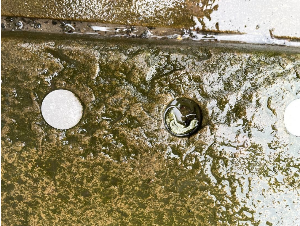
Photograph 7 – Missing nosing marker to entrance steps
