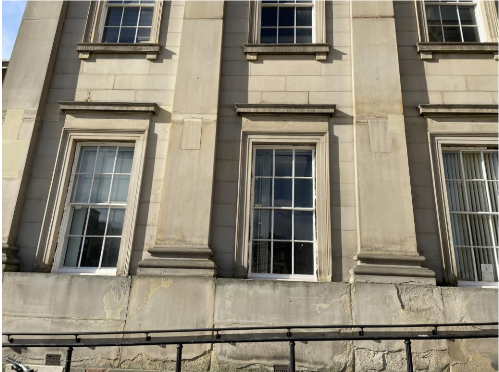
Photograph 11 – Areas of historic fixings to façade
