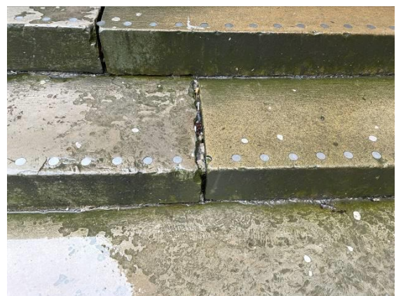
Image 17 – Mortar erosion to steps
