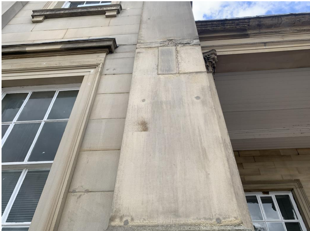
Photograph 11 – Areas of historic fixings to façade
