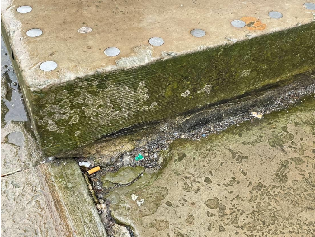
Photograph 5 – Build-up of debris between eroded mortar joints to steps
