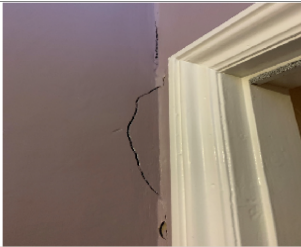
Photograph 5 – Cracking in the office – first floor adjacent to the landing
