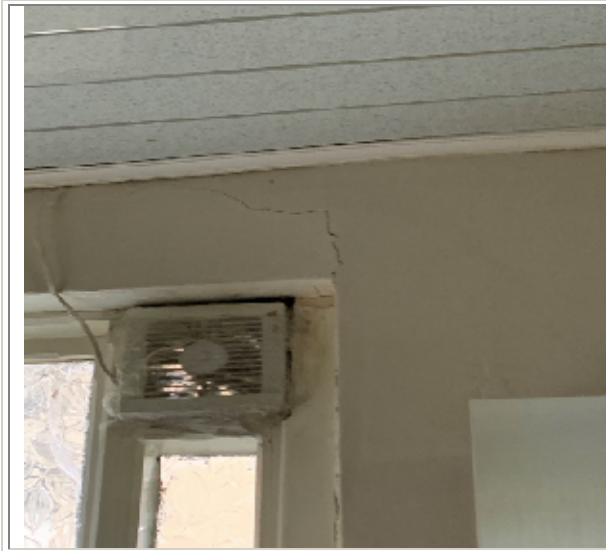
Photograph 7 – Cracking in the kitchen above the rear exit door
