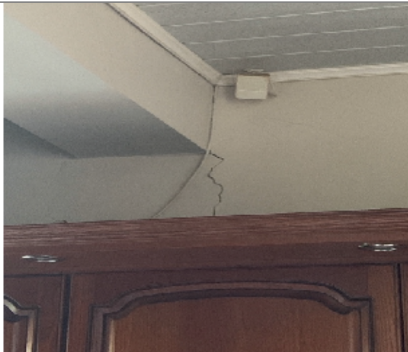
Photograph 6 – Cracking in the kitchen on the party wall
