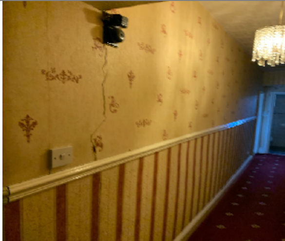
Photograph 4 – Cracking on the landing on the internal wall
