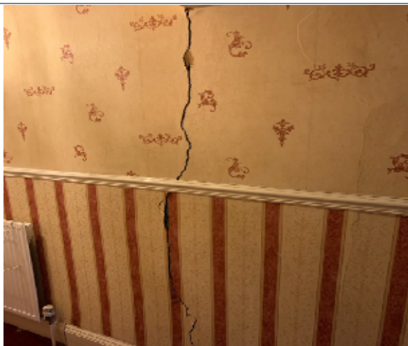
Photograph 3 – Cracking on the landing along the party wall
