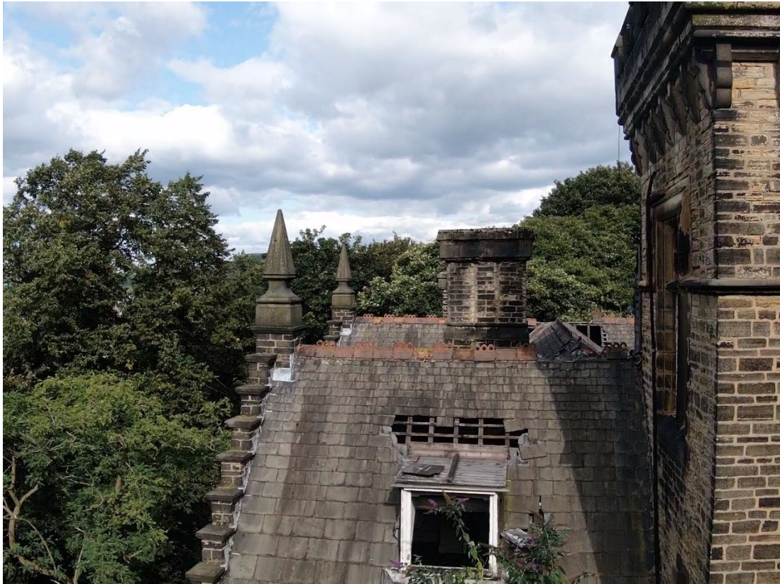
Photograph 6. The north-western aspect of B1 with gaps in the roof and a dormer window providing potential for roosting bats
