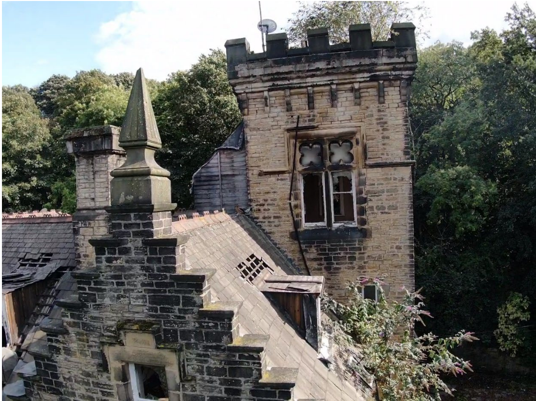
Photograph 8. Northern aspect of the tower and roof gaps.
