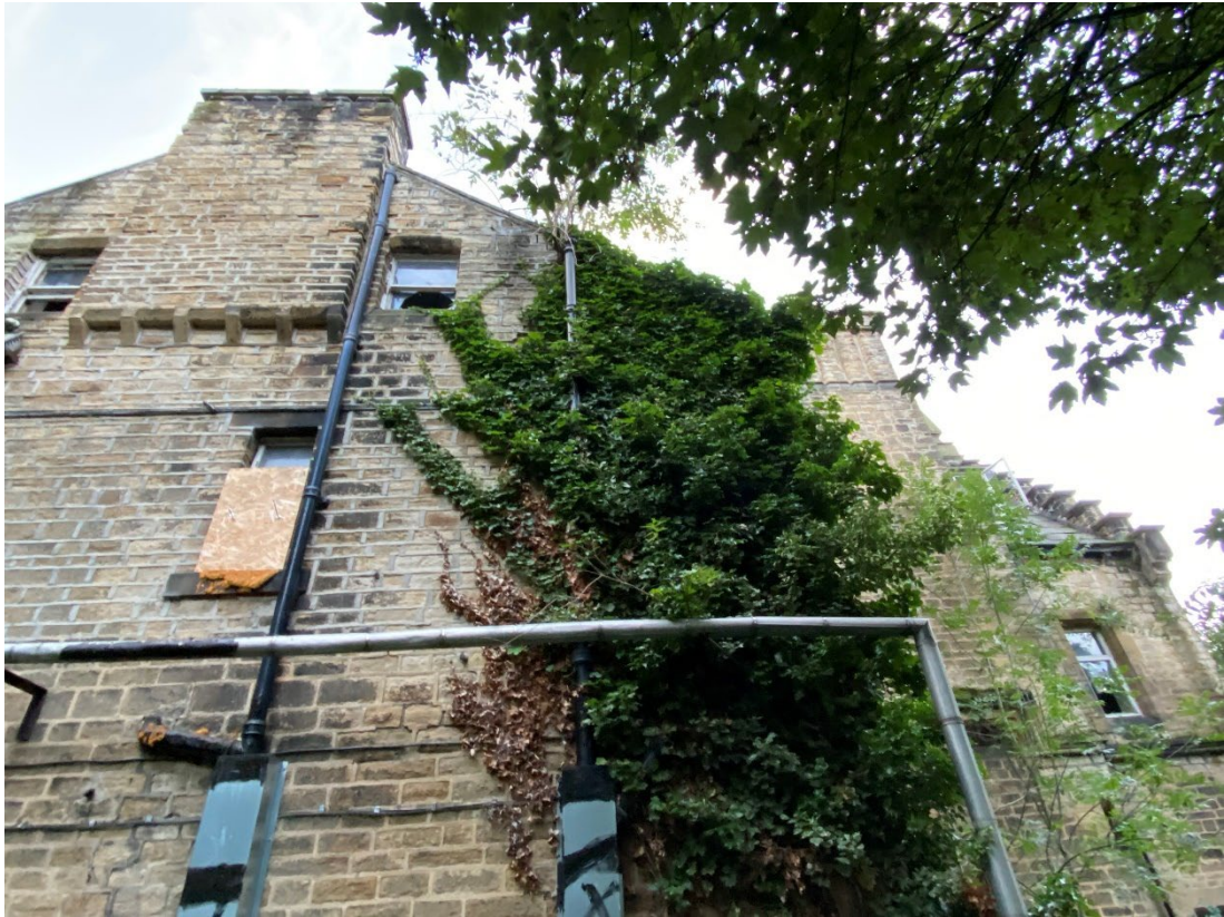
Photograph 4. Dense ivy coverage on the eastern aspect of B1
