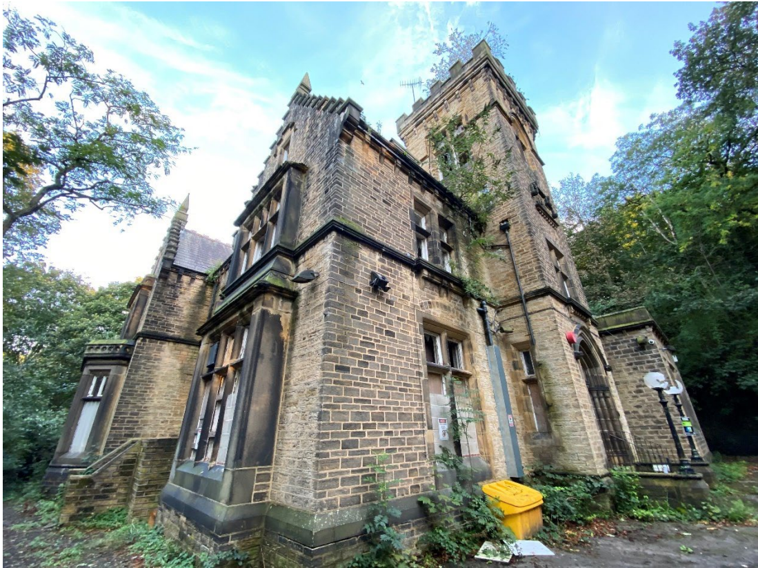
Photograph 2. The northern and western aspects of B1 with broken windows
