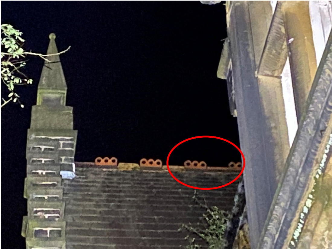
Photograph 10. Likely emergence location within ridge tile gap during emergence survey #3 (R2)
