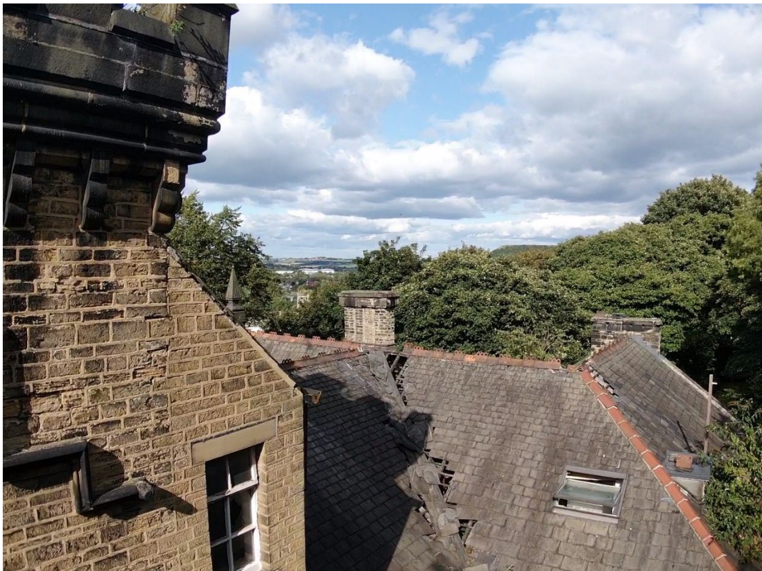
Photograph 7. B1, western aspect, damaged roof, and broken window.
