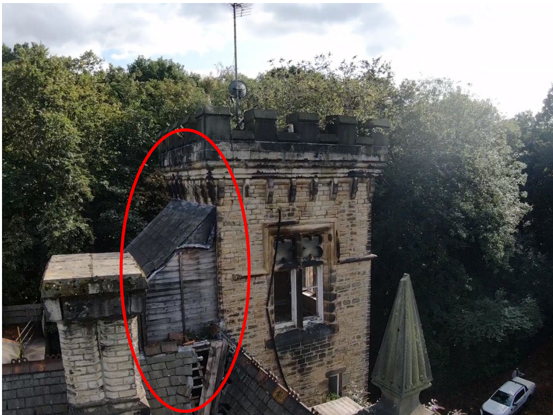
Photograph 9. The eastern aspect of the tower of B1. Likely emergence location for a bat during emergence survey #1 (R1).
