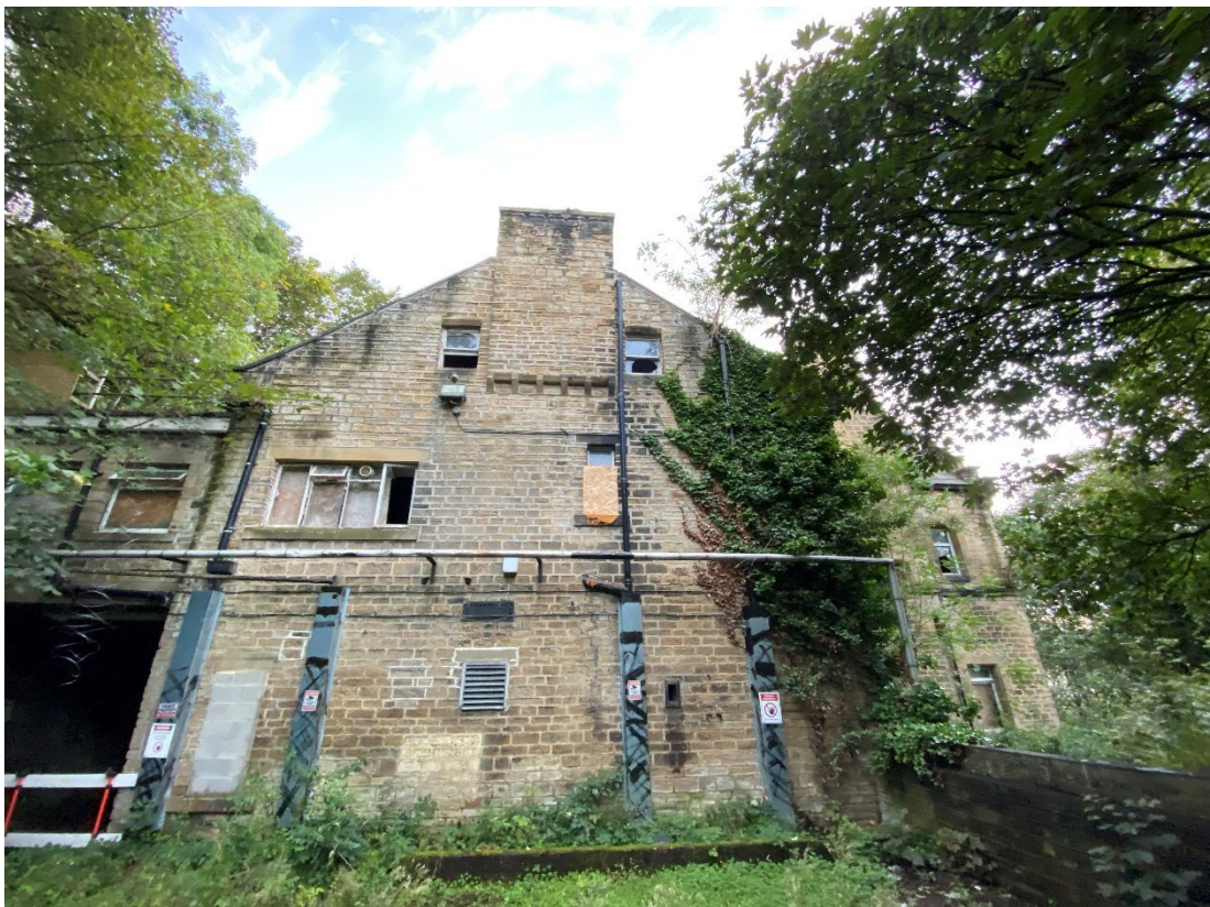
Photograph 3. The eastern aspect of B1 with good condition stone-work and broken windows
