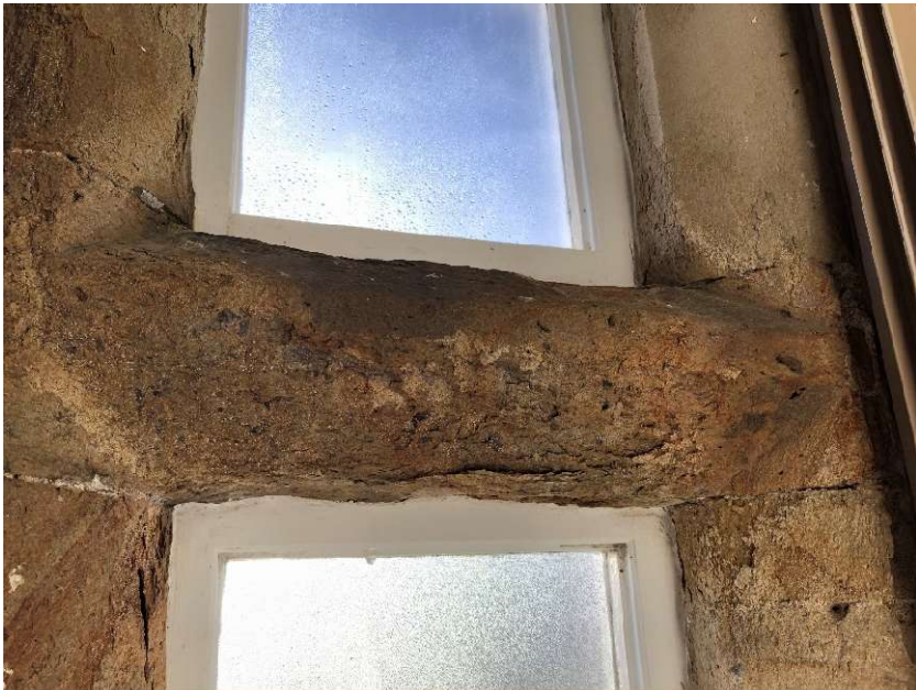
Internal view: Significant stone decay to the window surrounds on the south elevation (FF.03)
