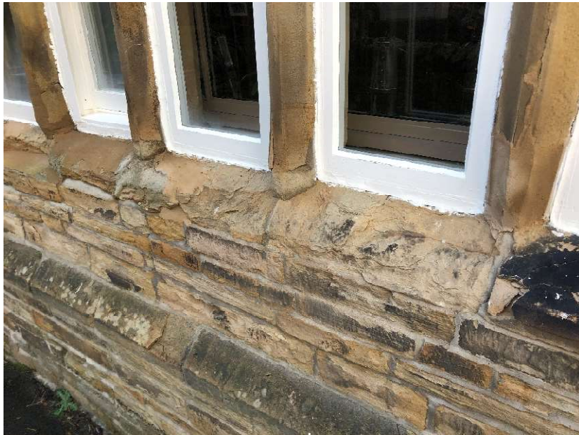
External view: Significant stone decay to the window surrounds on the south elevation (GF.04)
