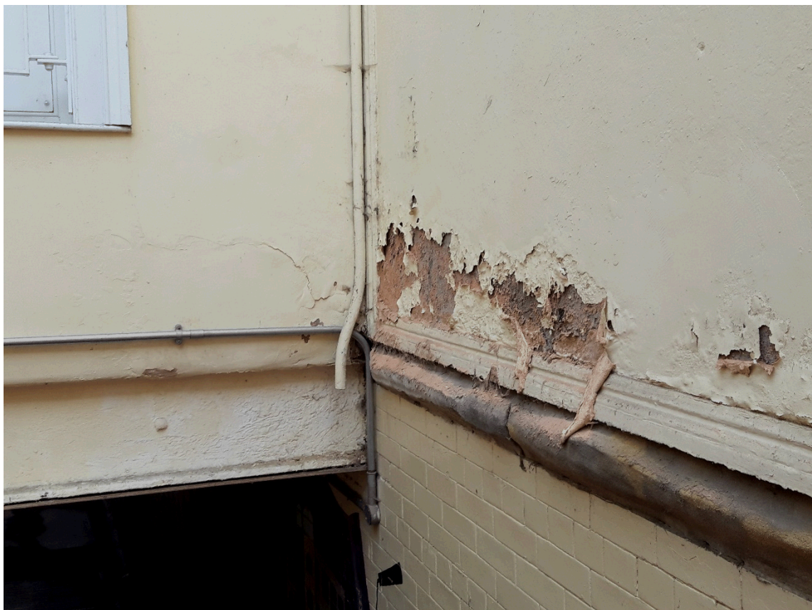
Insert 2-8 Close up of damage and evidence of water ingress on the walls.
