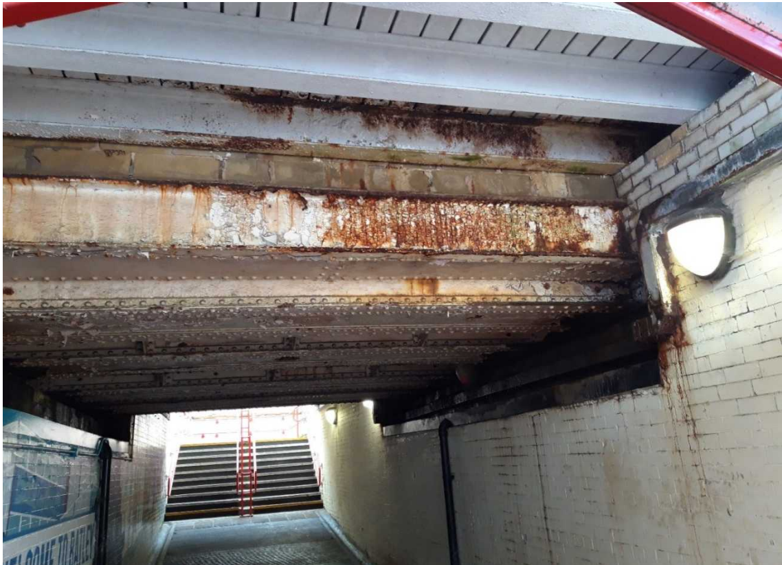
Insert 2-7 Batley Station Subway, showing the underside of the track deck. Note the poor condition and evidence of water ingress on the walls.
