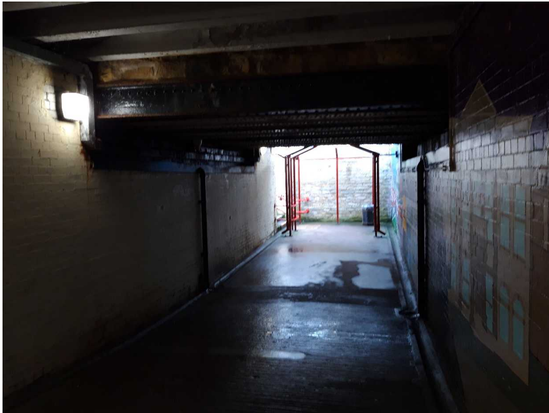
Insert 2-9 View from inside the subway showing dark and damp conditions.
