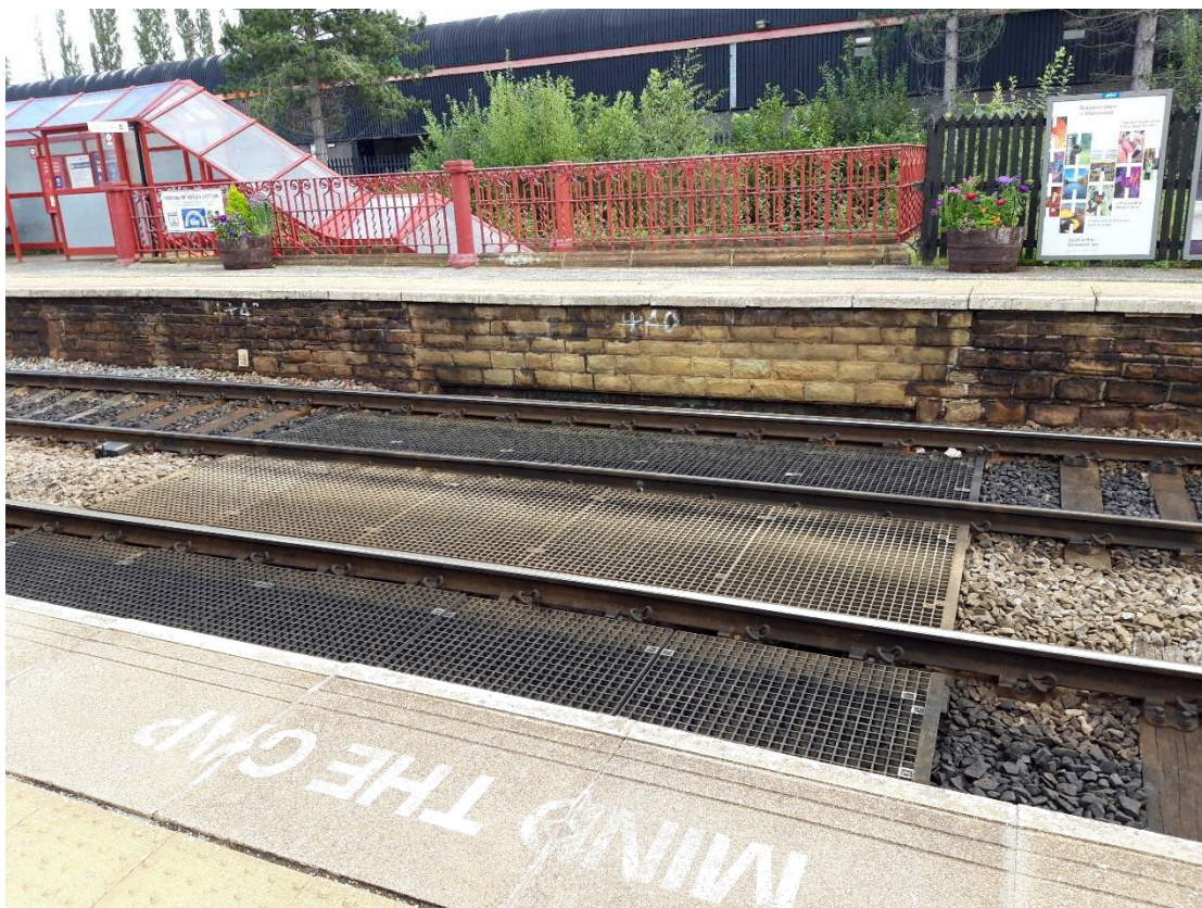
Insert 2-10 View of the section of rail tracks crossing over the subway.
