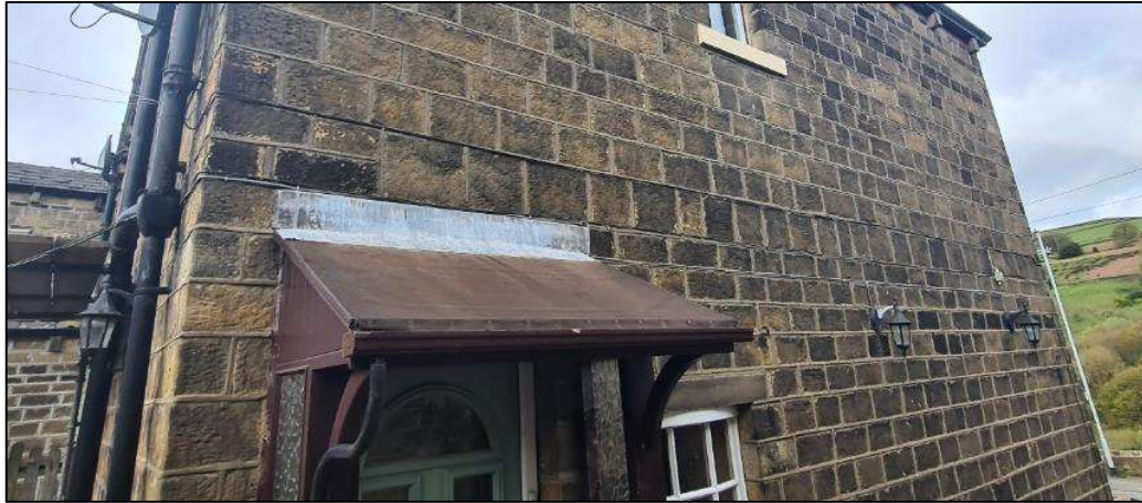
Plate 3. The eastern aspect of the building showing the building-mounted lamps
