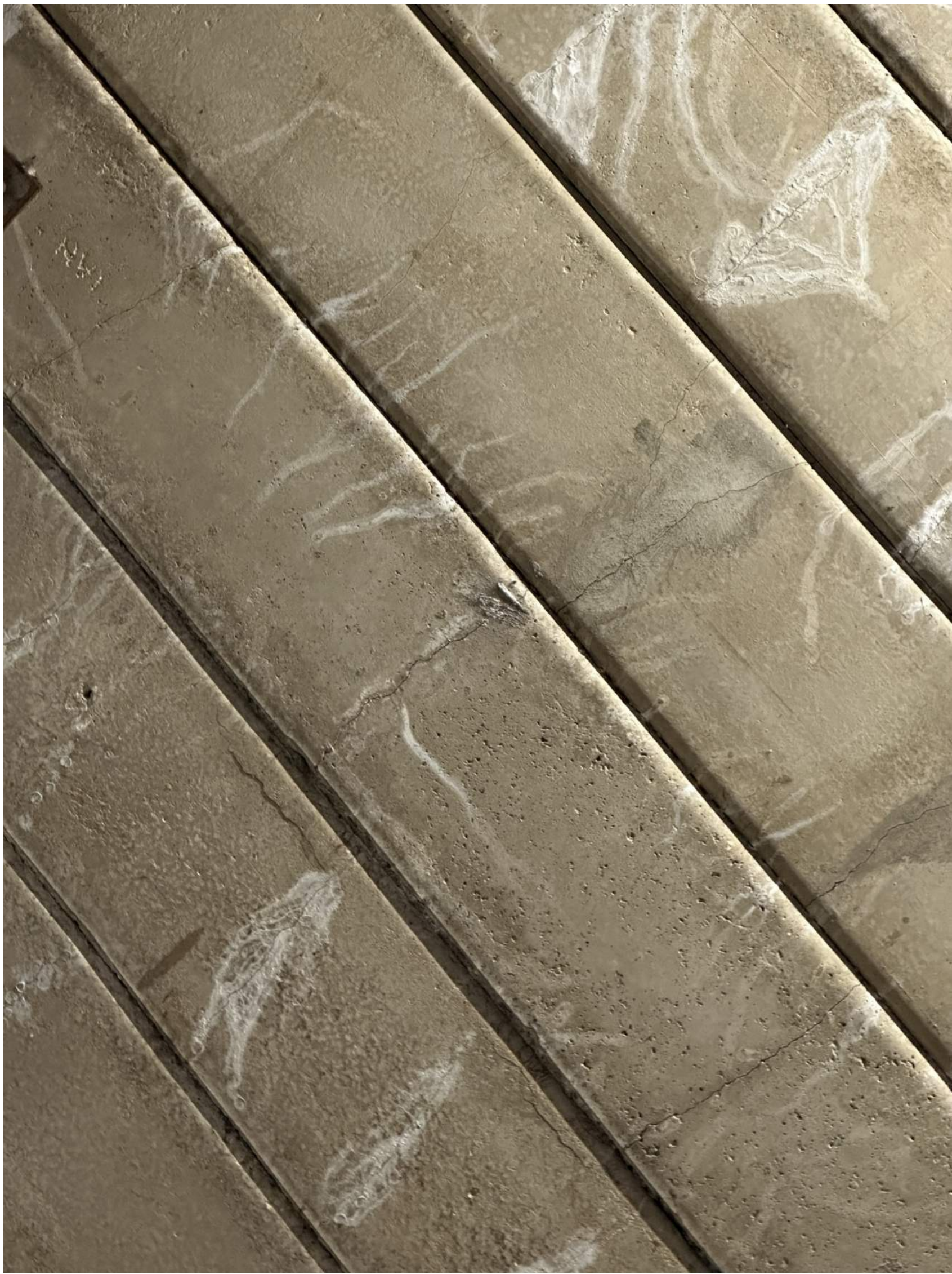
TYPE 2: MANY VISIBLE BENDING CRACKS (SIGNS OF WATER SEAPAGE MAY ALSO BE PRESENT AND/OR LARGE BENDING CRACKS) - EXAMPLE:
