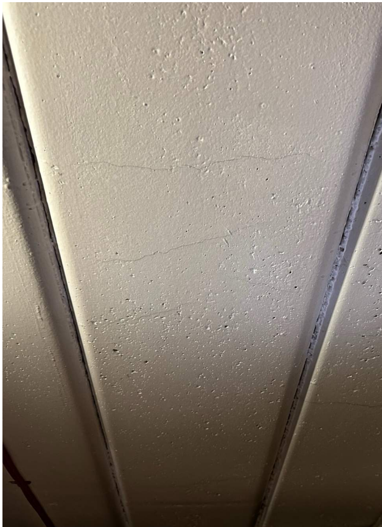
TYPE 1: VISUALLY IN GOOD CONDITION (SMALL BENDING CRACKS MAY BE PRESENT) - EXAMPLE:
