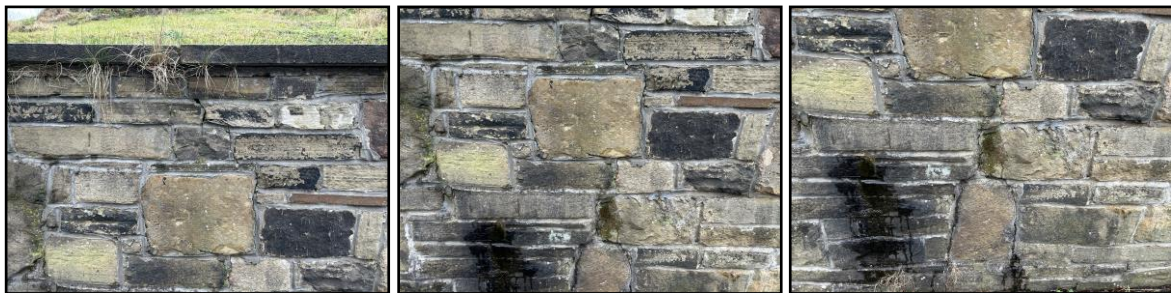
Crack 3 – 18.0m from top corner of wall
