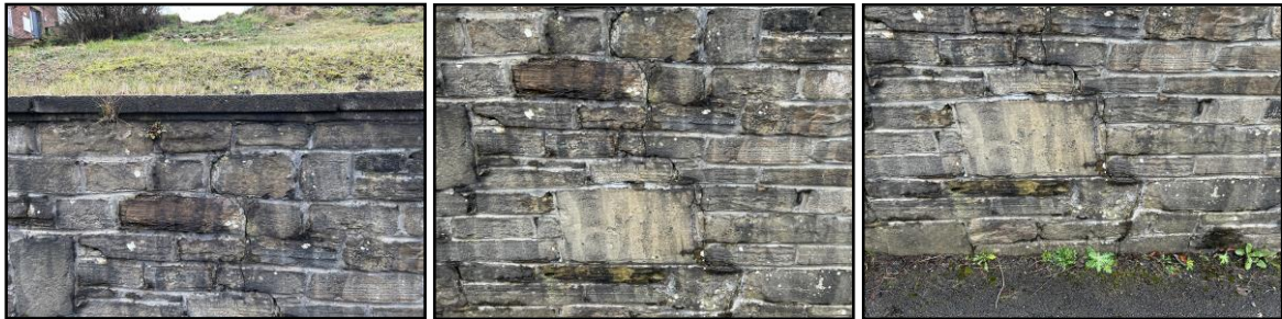
Crack 2 – 12.0m from top corner of wall
