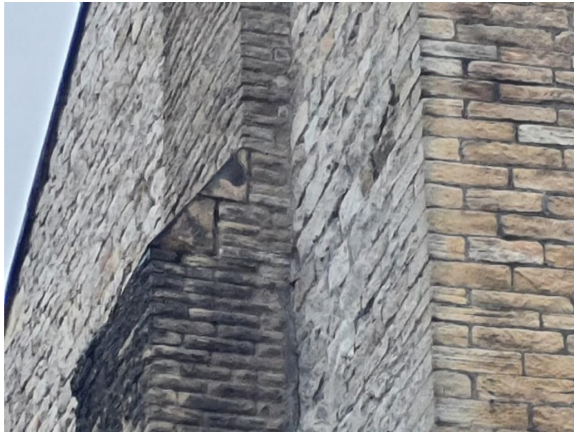
Figure 8 Showing weathering to mortar on AB1
