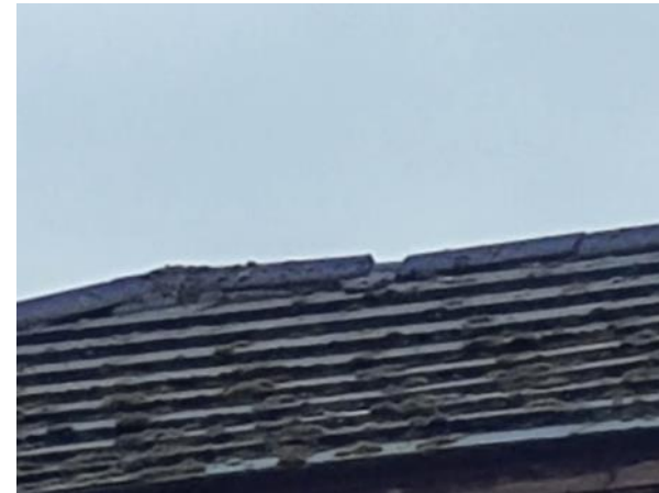
Figure 7 Showing gap to roof ridge
