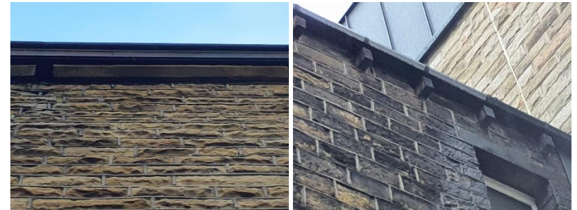
Figure 6 Showing gaps to cornice (l) and location of gap at eaves (r)
