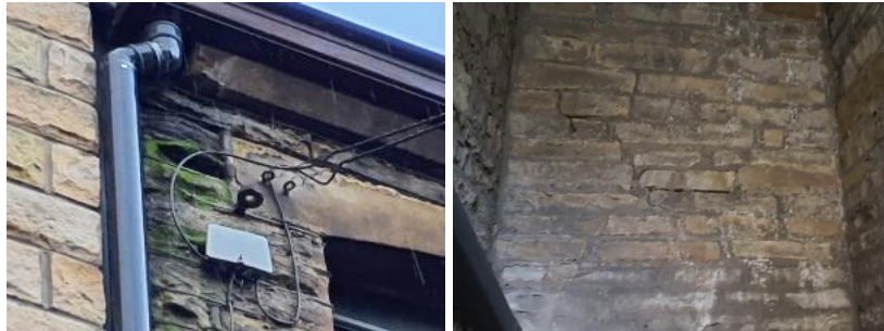
Figure 4 Showing hole on western elevation (l) and damaged passageway brickwork (r)
