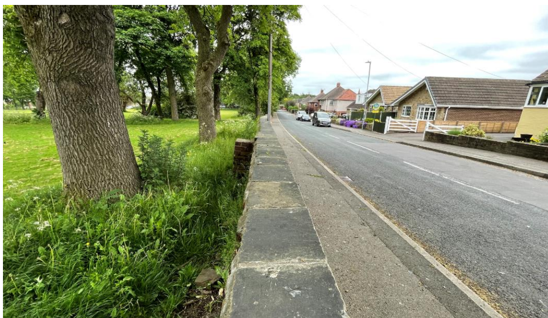
Photo 7 - Lack of perimeter fencing to West boundary of site off Sugar Lane.
