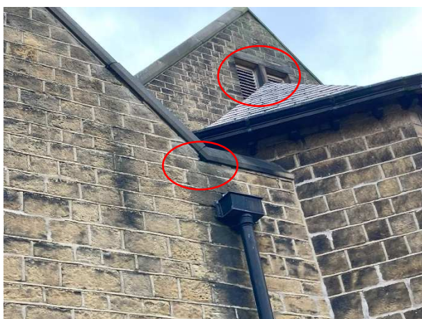
Photo 9: Missing mortar and air vent on the southern aspect, viewed from the southwest.
