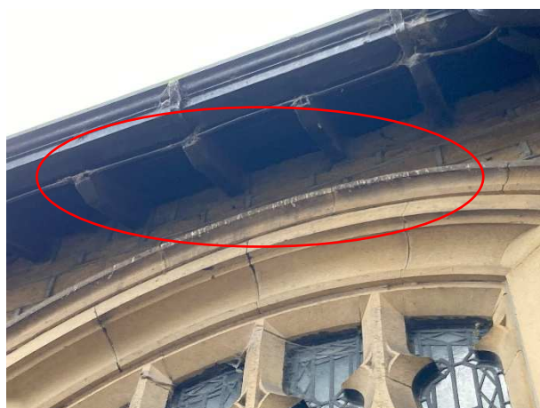
Photo 10: Gaps in the eave on the western aspect, viewed from the west.
