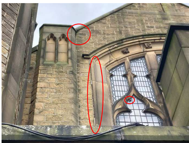
Photo 7: Missing mortar and broken window on the northern aspect, viewed from the north.
