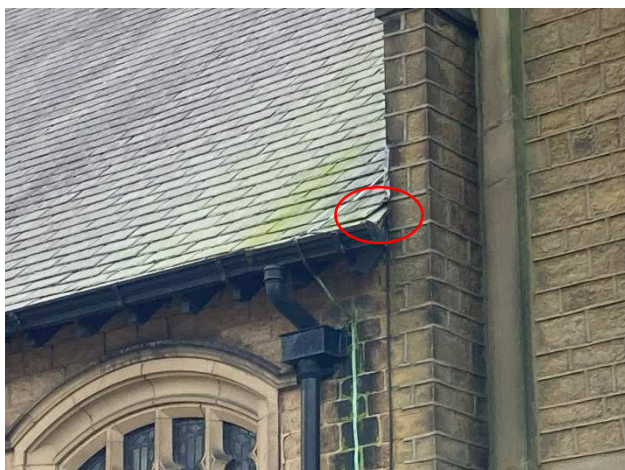
Photo 13: Lifted tile on the eastern aspect, viewed from the northeast.
