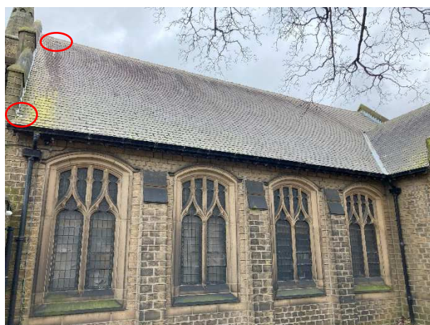
Photo 12: Missing tiles, on the western aspect, viewed from the west.
