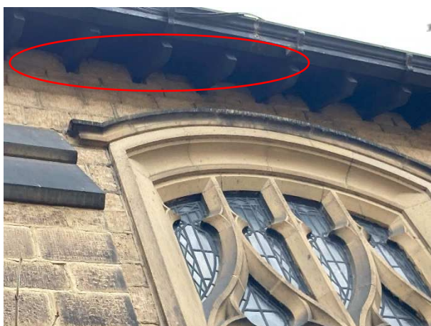
Photo 11: Gaps under the common rafters on the eastern aspect, viewed from the east.
