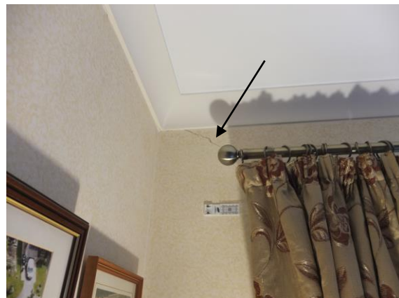
Internal crack to front left corner of rear mid-section dining room
