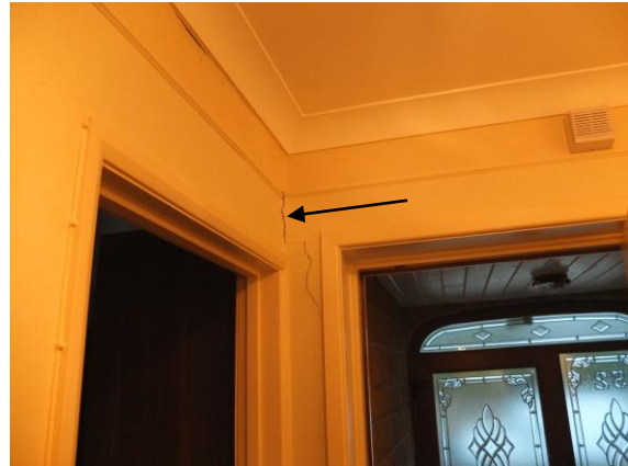
Internal crack to right of front entrance door leading to porch
