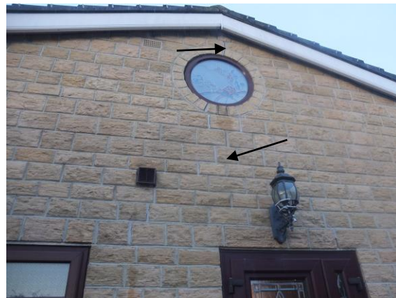
External cracking above rear kitchen door leading into high level roof
