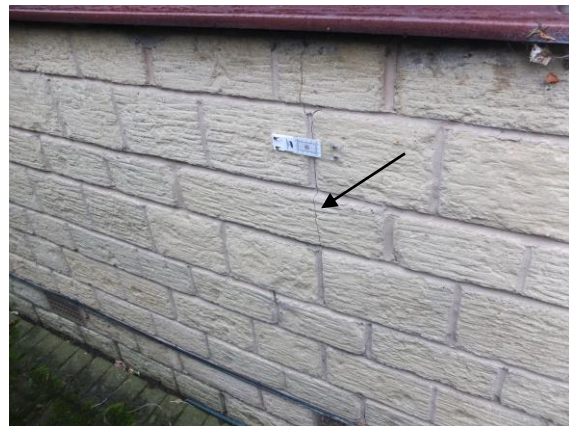
External crack beneath left mid-section dining room window
