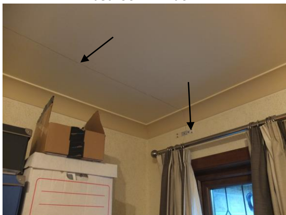
Internal cracking to front right to front mid-bedroom
