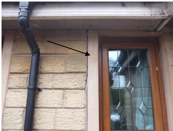
External cracking around concrete window reveal to left of front mid-section bedroom window
