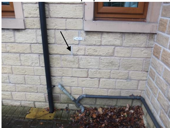
External cracking beneath front mid-section bedroom window
