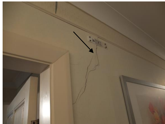
Internal cracking to rear wall of inner hallway to right of door leading to rear kitchen
