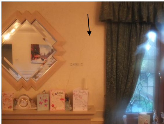
Internal crack to right of front left lounge chimney breast
