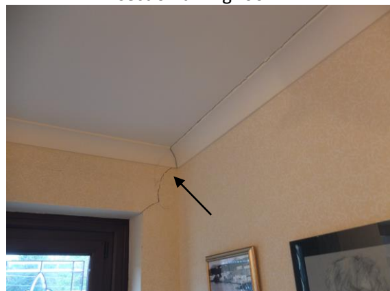
Internal cracking to right internal wall to rear kitchen
