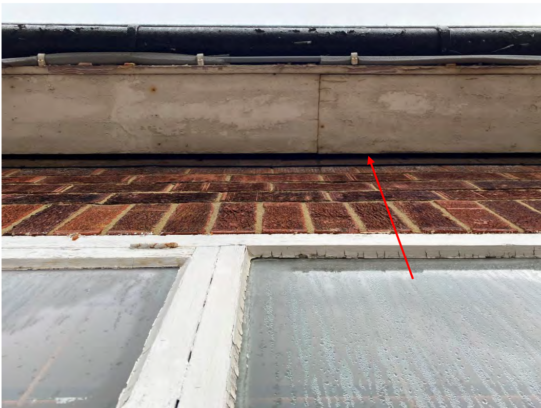
Photo 6. Potential bat roost feature at gap behind soffit on west elevation of on-site building (Jan 2023)
