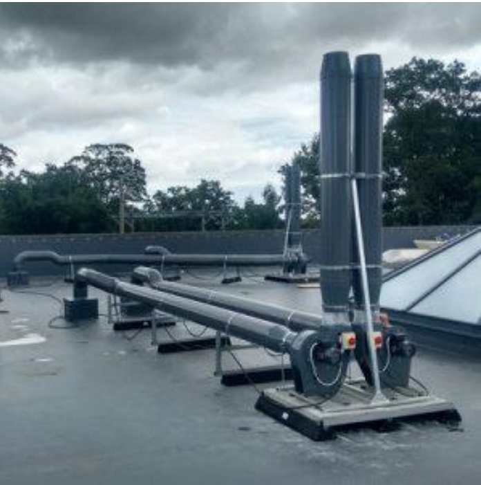
4.2.6 - Typical fume cupboard exhaust air roof fans
