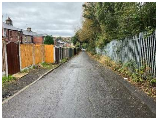
Photo 11 – Trench scars for length of carriageway, overgrown vegetation on edges of footway and carriageway. Leaf deposits on both sides of carriageway.
