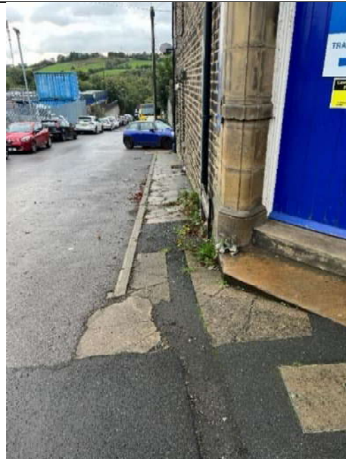
Photo 2 – Footway severely fatigued, visible trench lines
