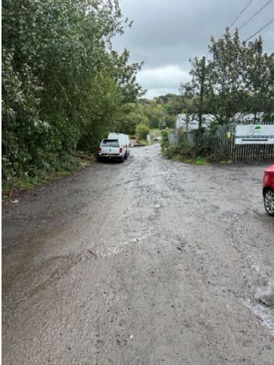
Photo 17 – Severely deteriorated carriageway surfacing
