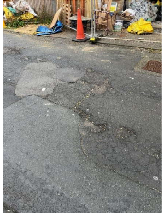
Photo 10 – Carriageway has deteriorated severely
