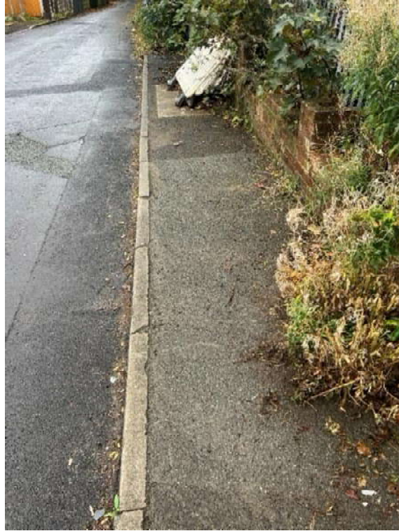
Photo 3 – Kerbing is chipped
