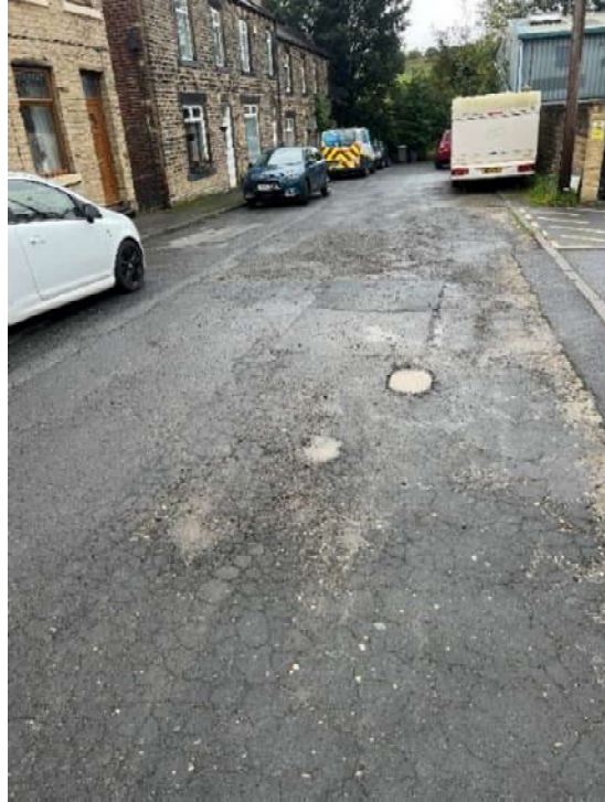
Photo 13 – Deterioration of carriageway, causing pot holes, pooling of water.
