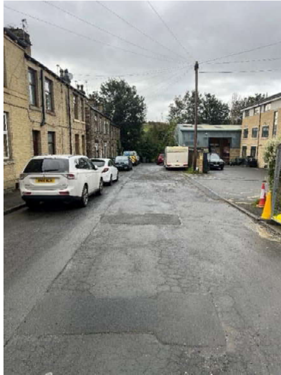
Photo 11 – Carriageway surfacing is fatigued and visible trench scars
