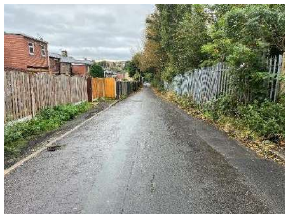
Photo 8 – Trench scars on surfacing full length of carriageway. General wear of carriageway.
