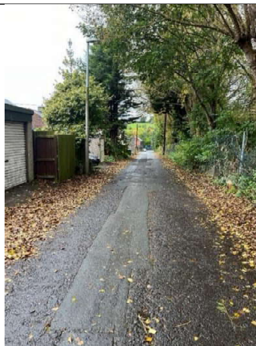
Photo 14 – Trench scars and deterioration of carriageway surfacing, leaf deposits on either side of carriageway.
