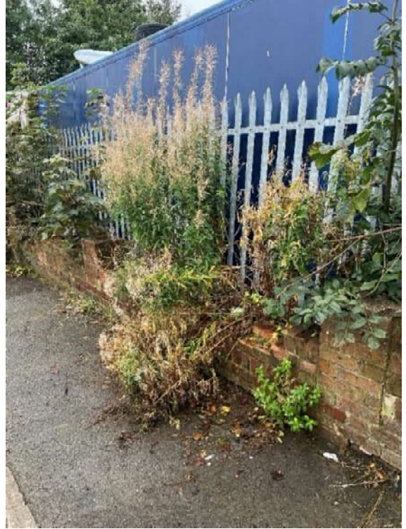
Photo 4 – Damaged brick work, over grown vegetation
