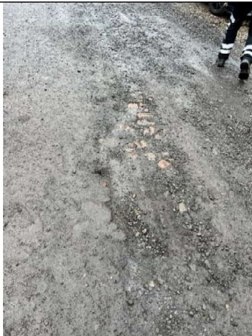
Photo 15 – Brick under surface exposed
