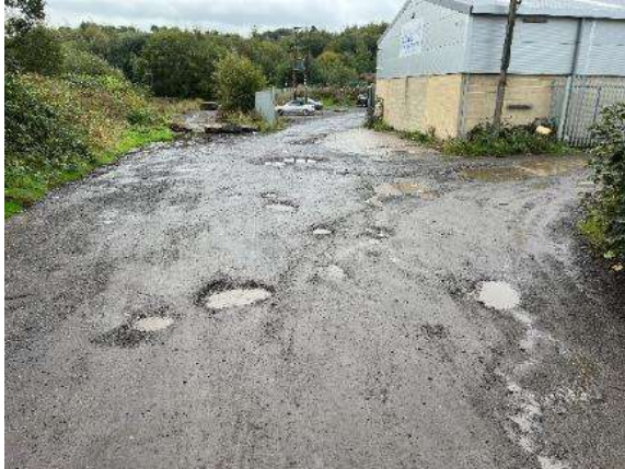
Photo 19 – Severe pot holes at bottom of street, with pooling of water.
