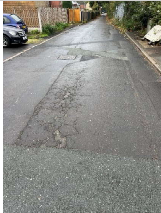
Photo 2 – Deterioration of carriageway surface, clear trench scars throughout the street
