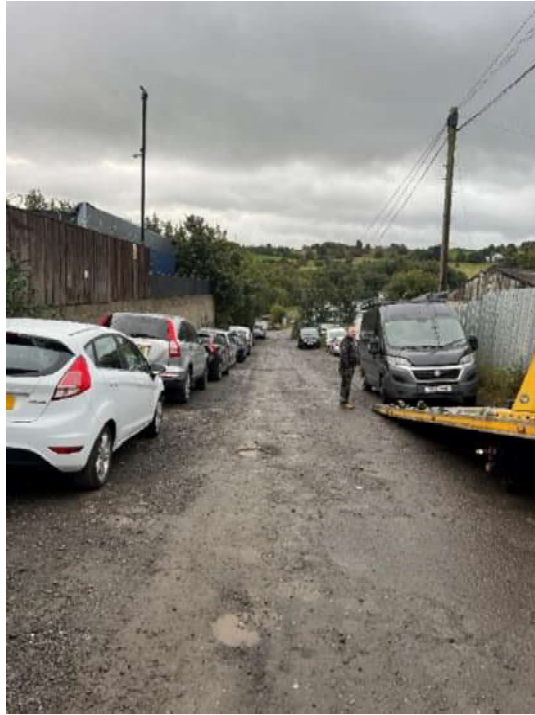
Photo 13 – Severely deteriorated surfacing, pitting and pooling of water.
