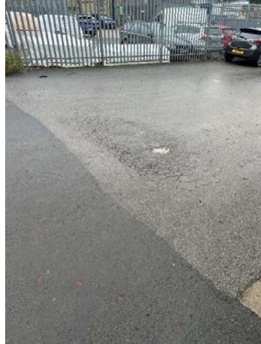
Photo 4 – Fatigued surface with water pooling in centre
