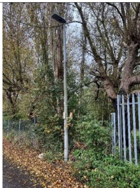
Photo 12 – Lighting column is slanted
