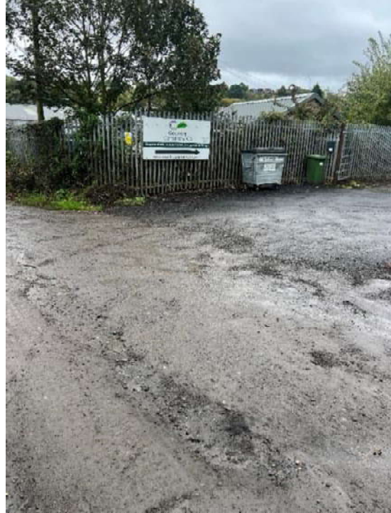
Photo 18 – Severely deteriorated carriageway surfacing
