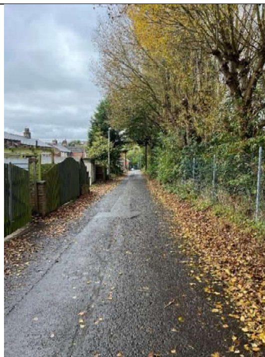
Photo 13 – Trench scars and deterioration of carriageway surfacing, leaf deposits on either side of carriageway.
