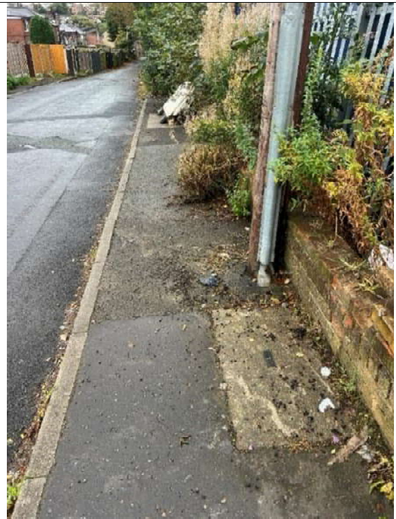
Photo 6 – Debris deposits on footway, scars on footway surfacing. Cover is in an acceptable condition. Kerbing is in acceptable condition.
