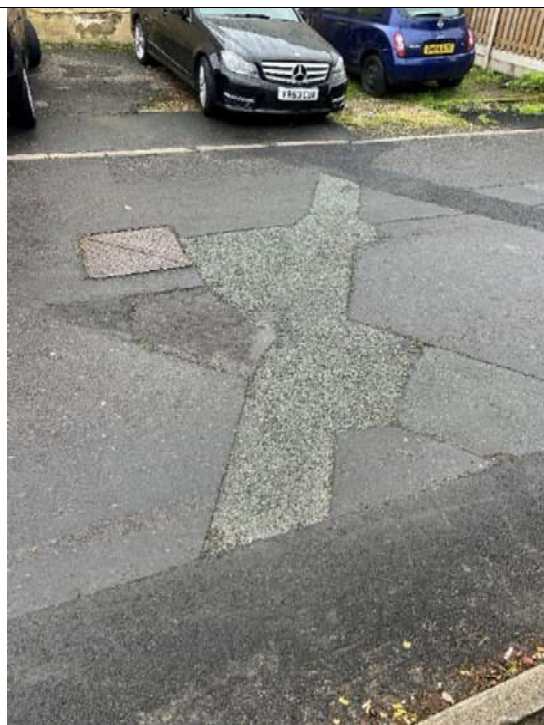
Photo 7 – Trench scars on carriageway surfacing. Iron works in acceptable condition. Debris deposits on kerbside. Kerbing on opposite side of road damaged and out of place.
