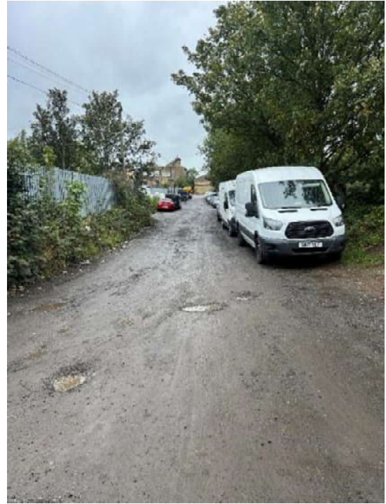
Photo 20 – Severe pot holes at bottom of street, with pooling of water.
