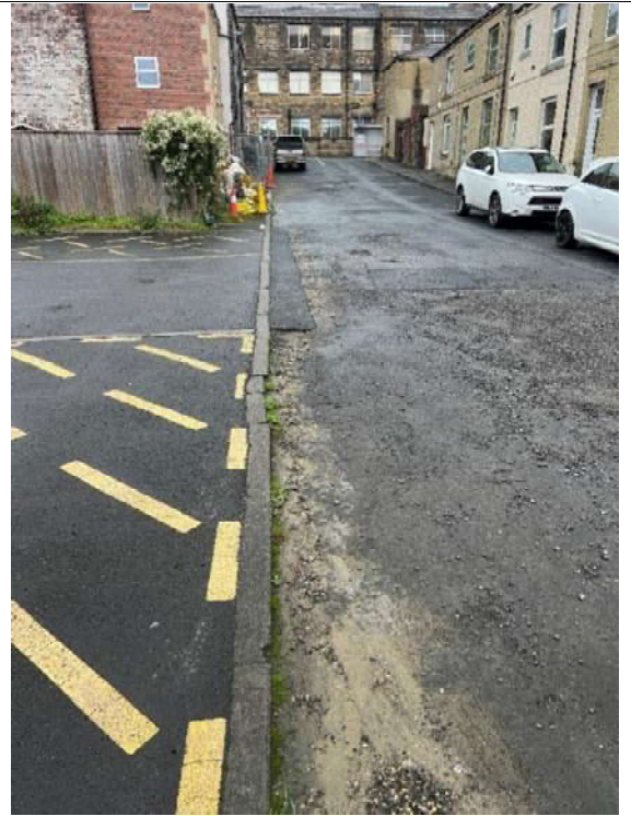
Photo 16 – Kerbing is out of place
