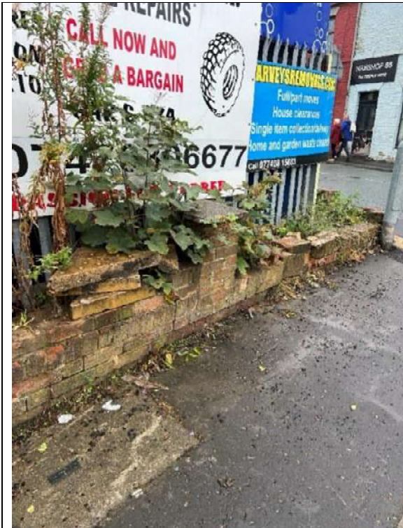
Photo 5 – Damaged brick work, overgrown vegetation
