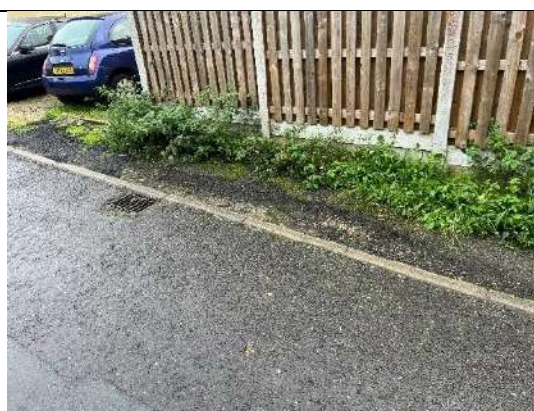
Photo 10 – Severely deteriorated footway surfacing, overgrown vegetation.
