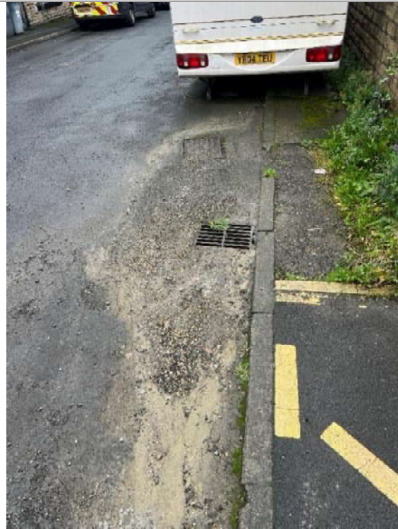
Photo 15 – Deposits around gully and cover. Gully is not blocked. Kerbing is cracked and damaged. Carriageway surface is fatigued.
