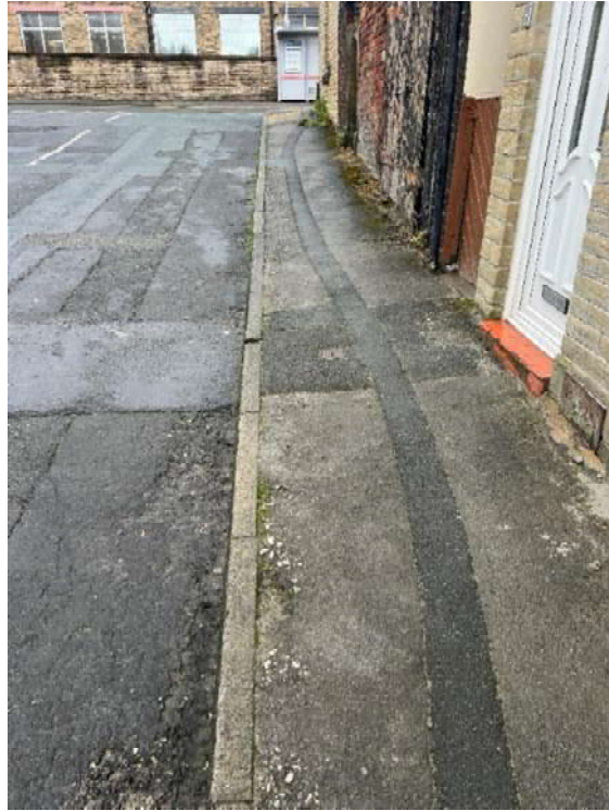
Photo 9 – Footway and carriageway severely fatigued along kerb line and visible trench scars in footway and carriageway.
