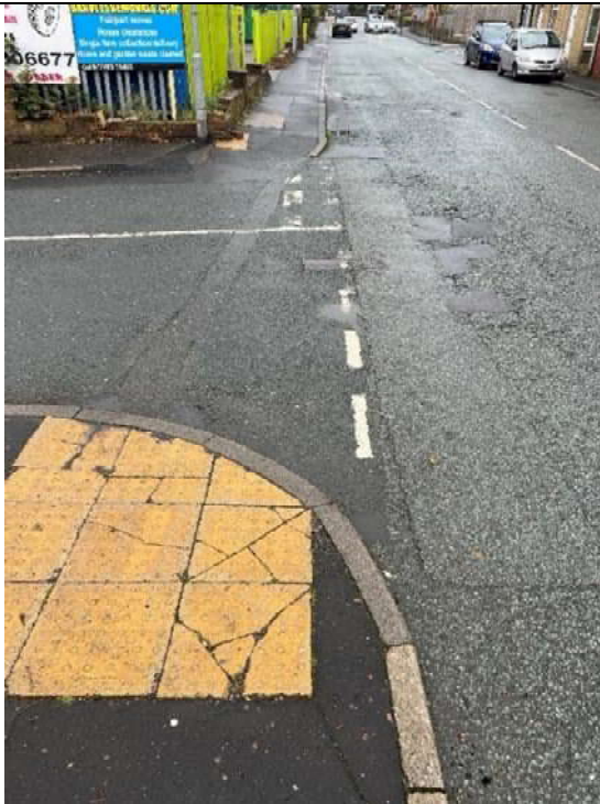
Photo 1 – Trench scars across the junction, junction markings worn, tactiles cracked
