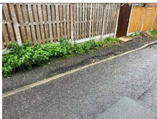
Photo 9 - Severely deteriorated footway surfacing, overgrown vegetation.
